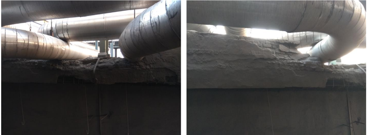
Interference of steam lines with bunker roof and parapet wall
