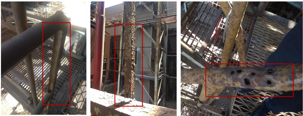
Corroded boilers structure and hand rails at different locations
