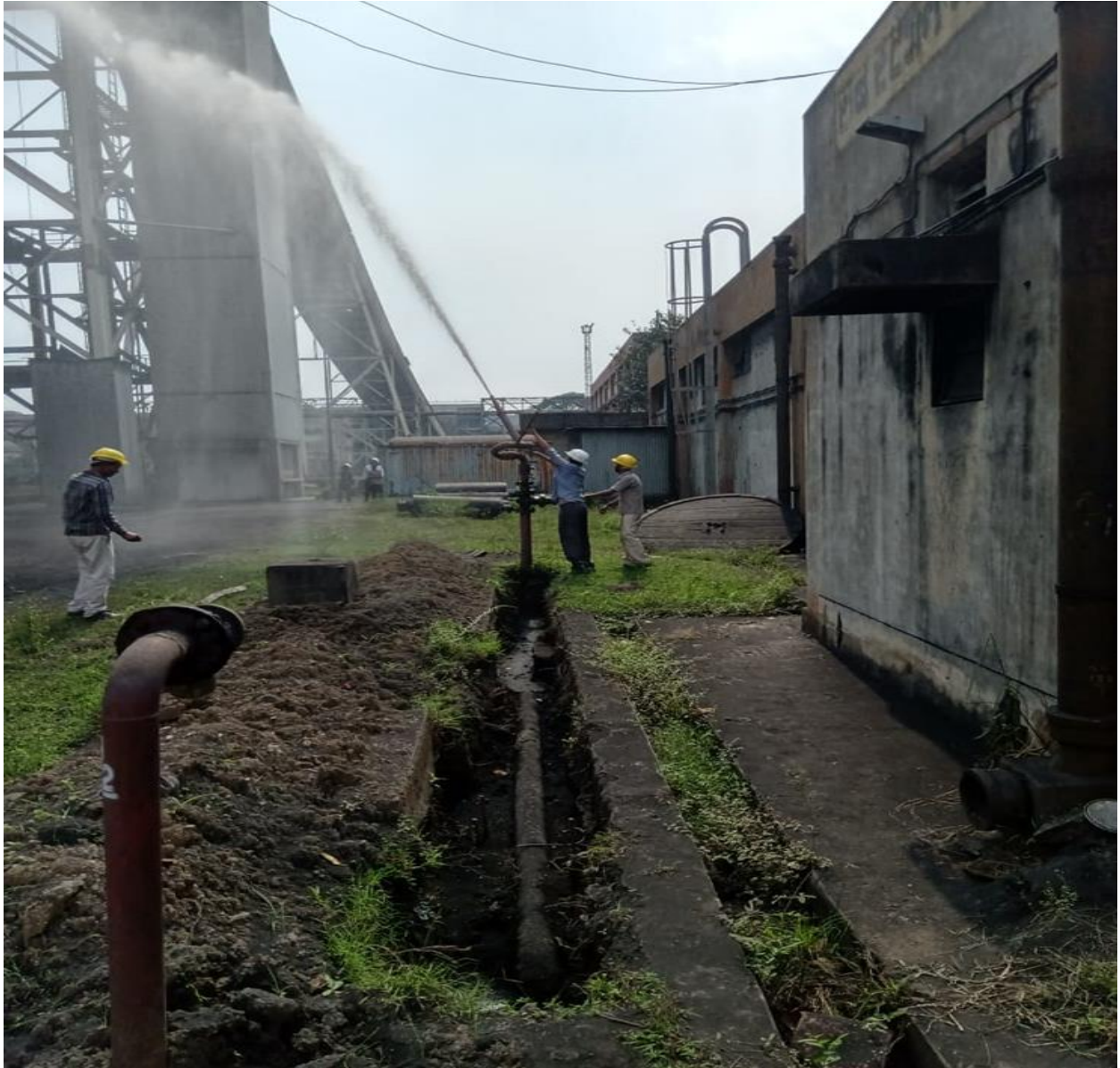
Testing of Fire Hydrant Pressure in Boiler Area at one of the TPS during Safety Audit
