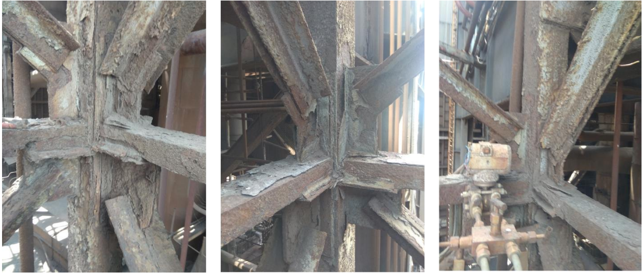
Corroded boilers structure at different locations
