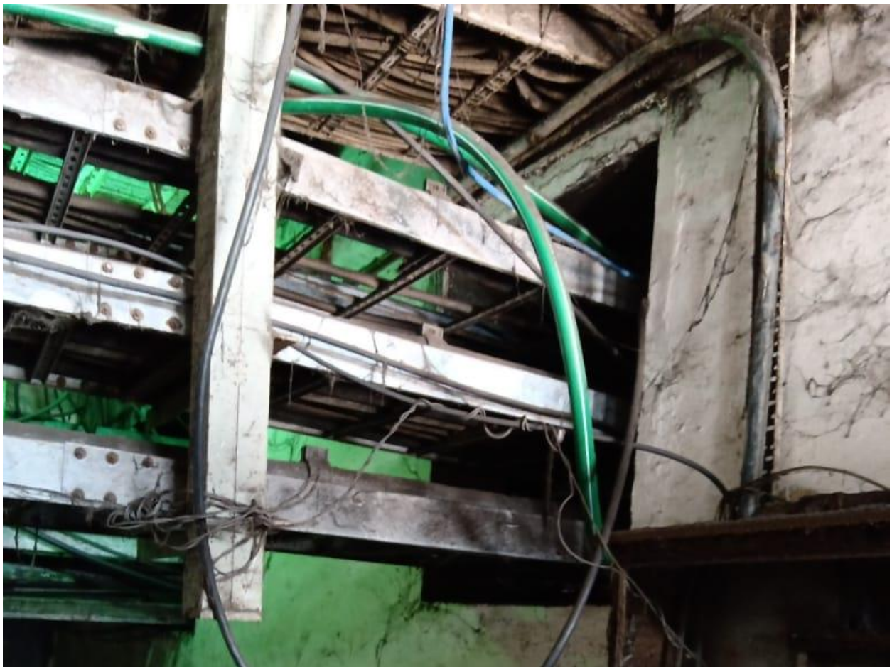
Improper Sealing of Cables at entry/exit
