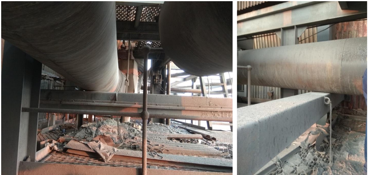
Interference of Steam line with LRSB
