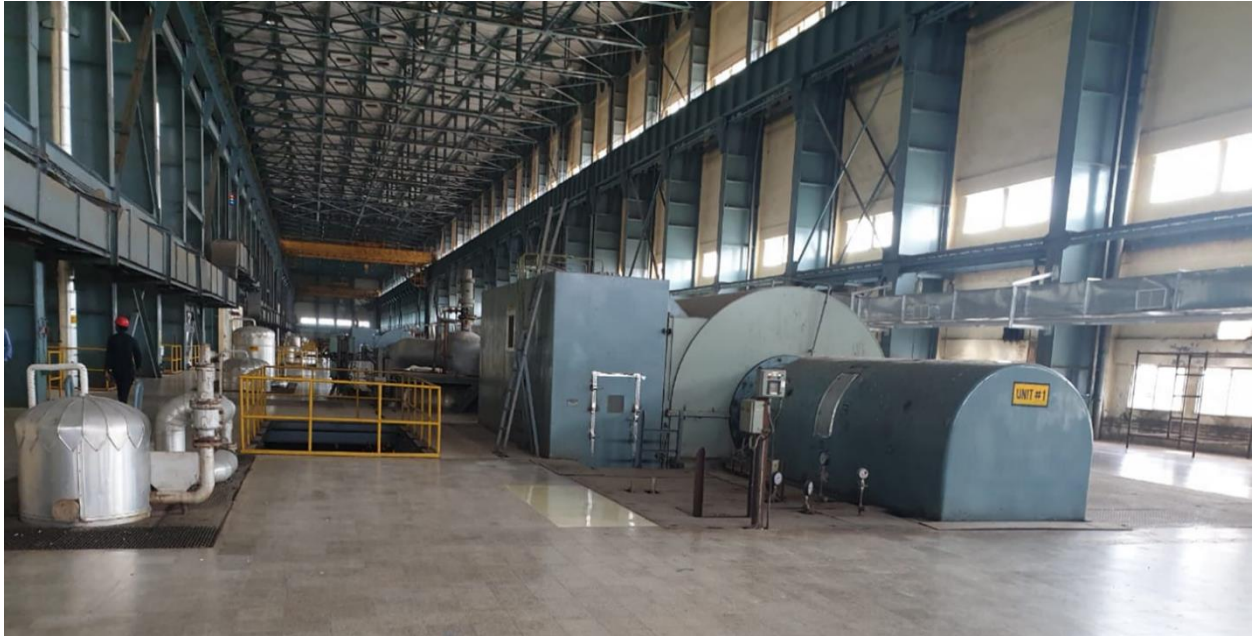
Well maintained Turbine-Generator floor of one of the TPS
