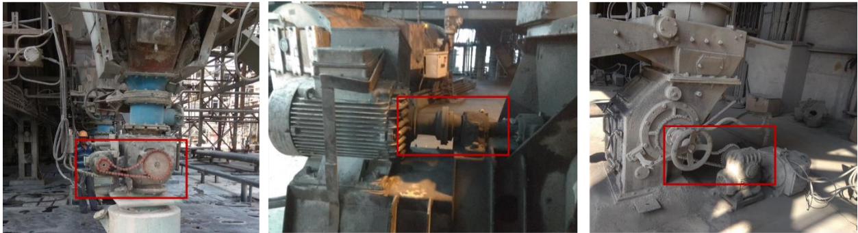
Rotating equipment without guard
