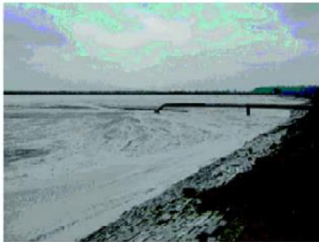
b) Safe Disposal for Control of Fugitive Dust with Uniform Discharge and Free Board
