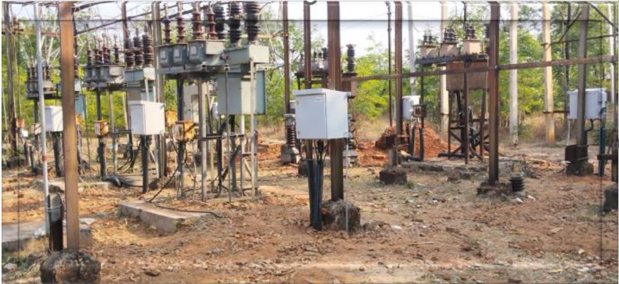
Figure 9. Complete substation with micro-CRP's
