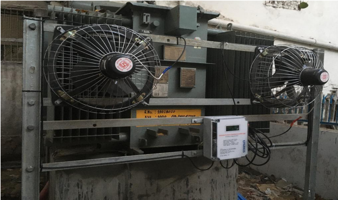
Plinth mounted DT with auto cooling system
