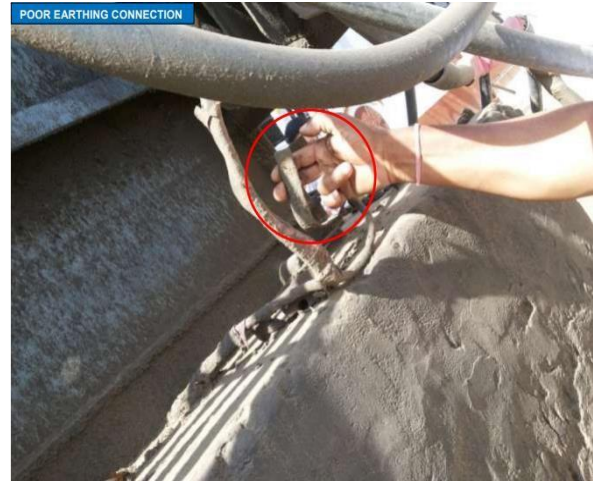
Figure 10: Improper rating of earth wire
