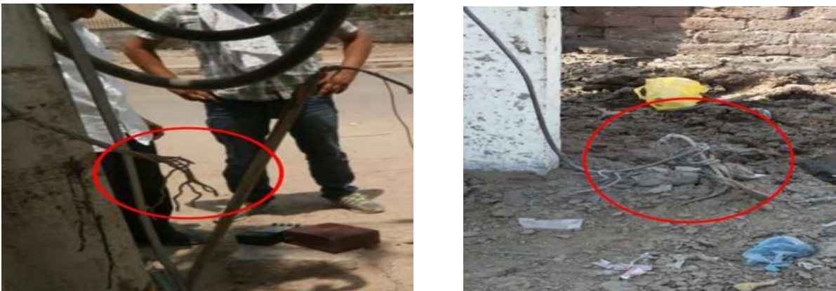
Figure 9: Improper Earthing Connection
