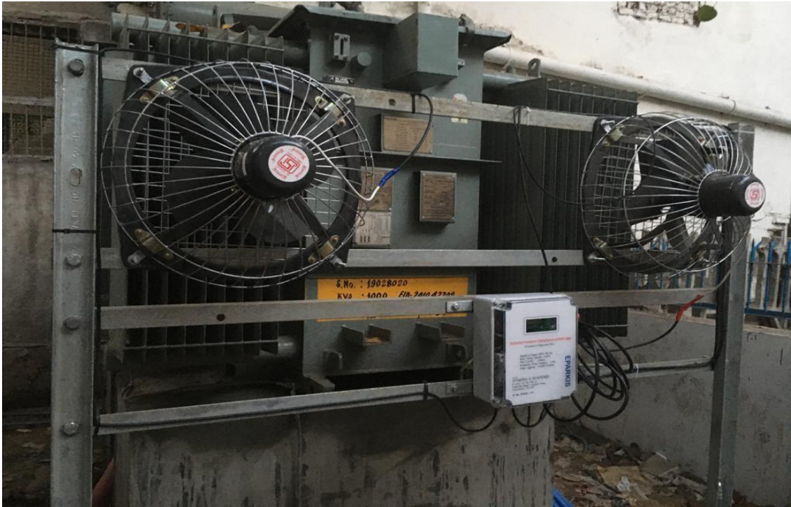
Plinth mounted DT with auto cooling system
