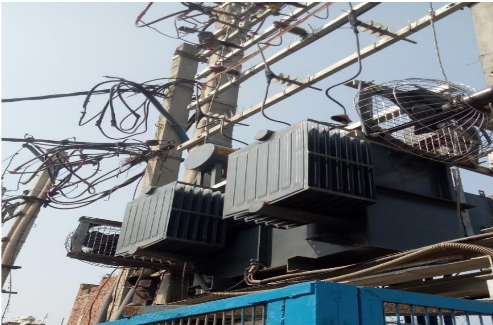
Pole mounted DT with auto cooling system
