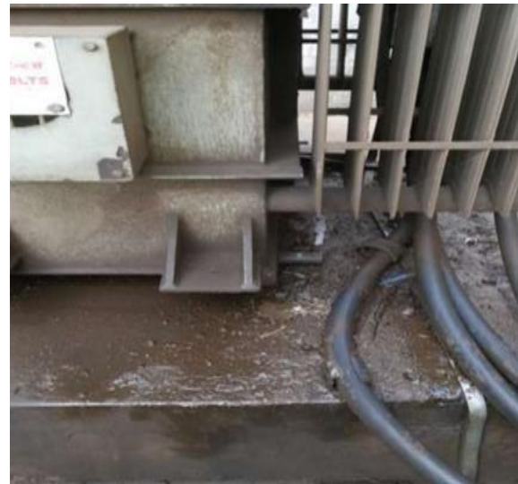
Figure 12: Heavy Oil Leakage
