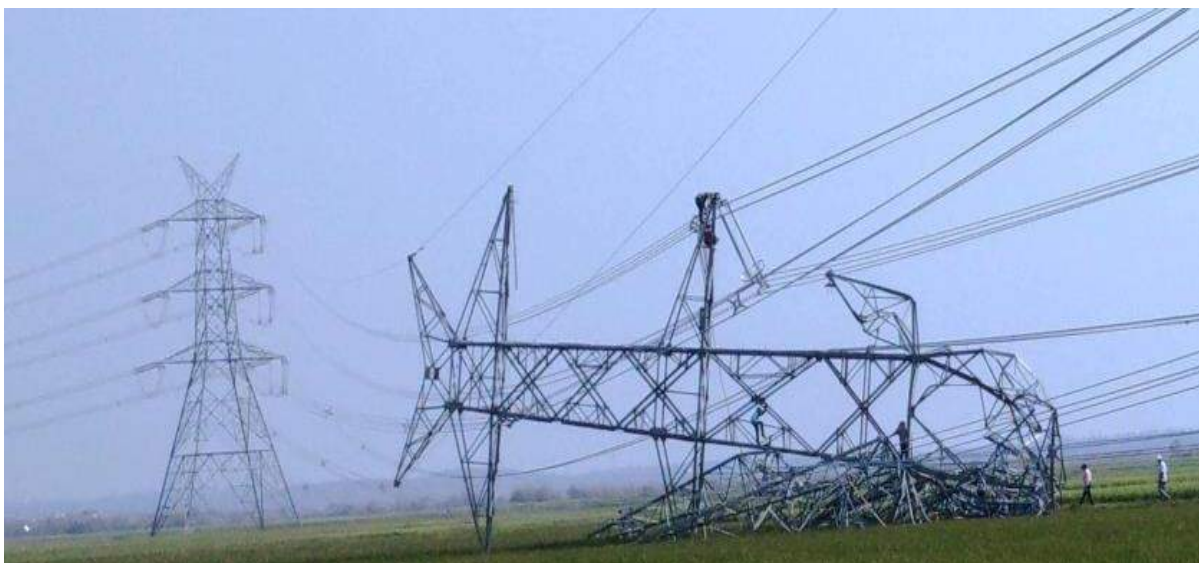
Tower at location no 15/1
