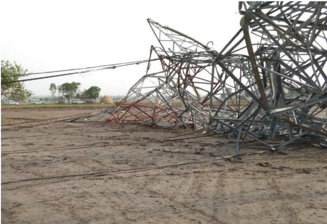
Tower at location no 59
