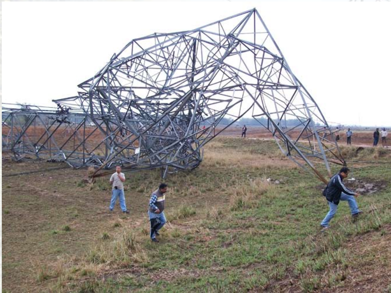
Inspection of Tower Failure
