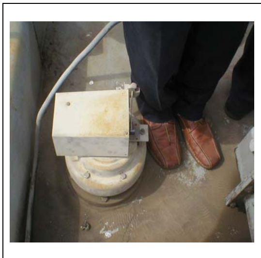
Exhibit-9 Clearly visible non operation of PRD
