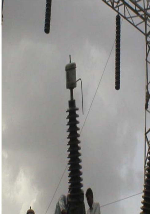
Exhibit-3 Popped up R –phase of HV bushing
