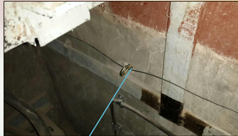
The LHD system sensor tube installed in one of the cable trenches in GAIL
