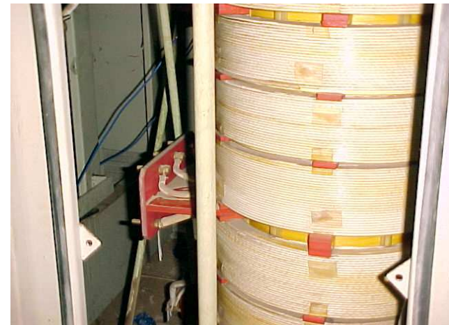
Status of windings of OVDT transformers after 72 hours in water (Worked perfectly fine just after drying)
