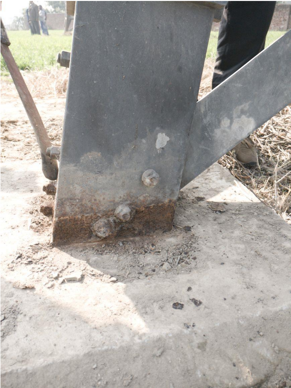
Fig. 6.1. Corroded leg of tower
