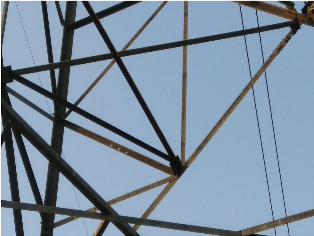
Fig. 3.3. Unplugged holes observed at Dadri Panipat Line (tower No. 274 A)
