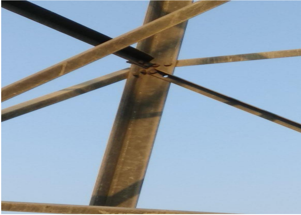
Fig. 3.2. Unplugged holes observed at Dadri Panipat Line (tower No. 274 A)
