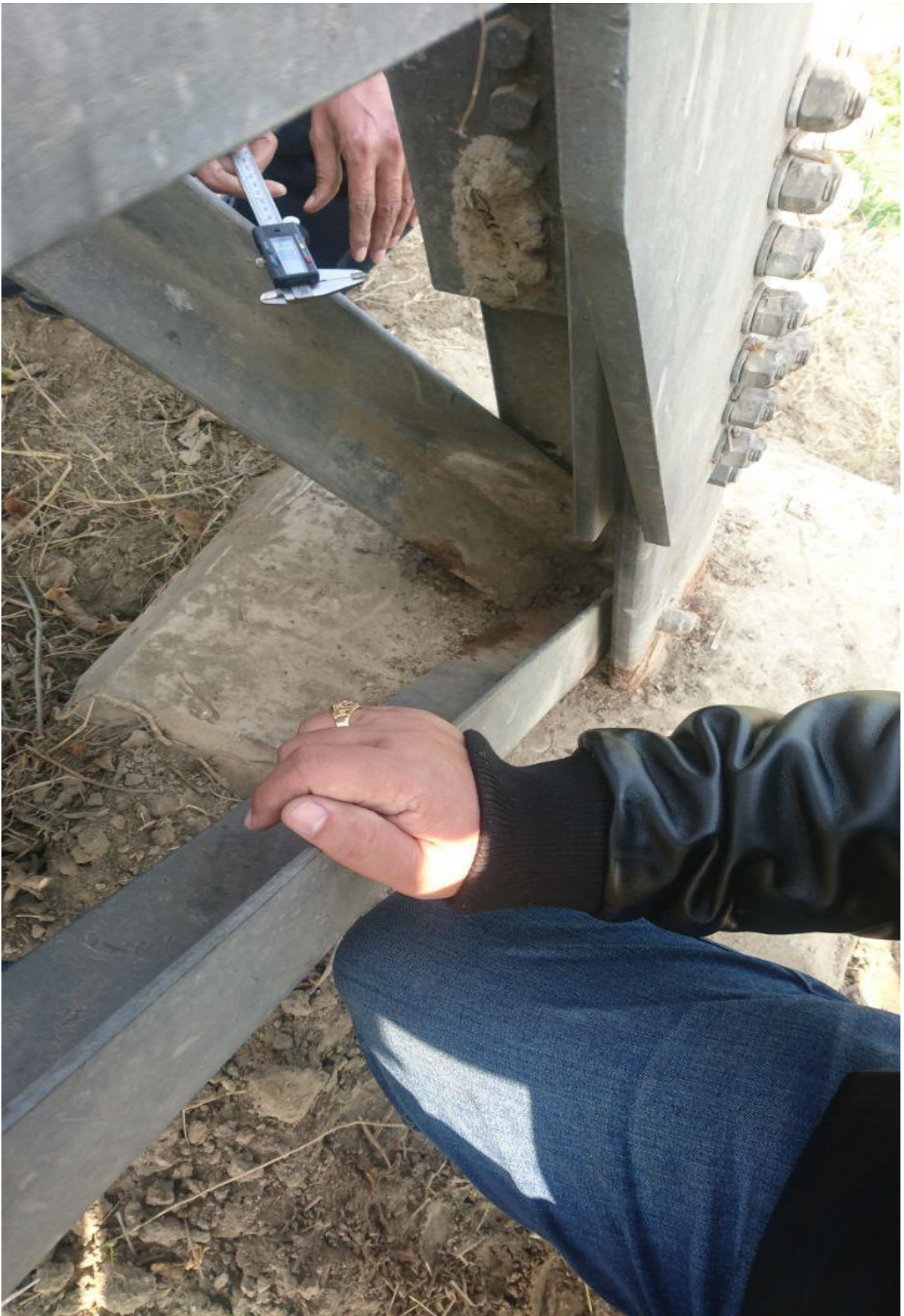
Fig. 6.2. Corroded member of tower
