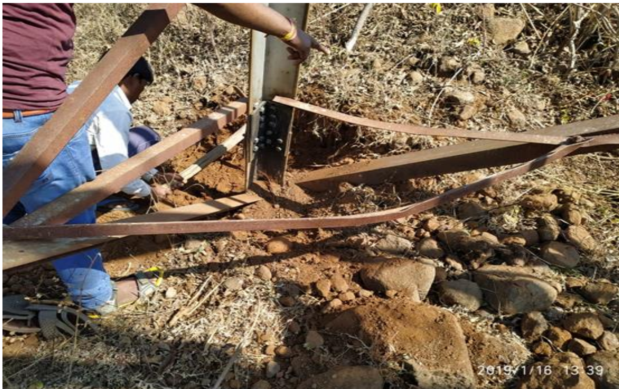
Figure 2. Bent, Buckled Members
