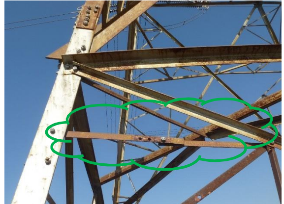
2.d) Rectification with two member pieces connected with single bolt on one flange
