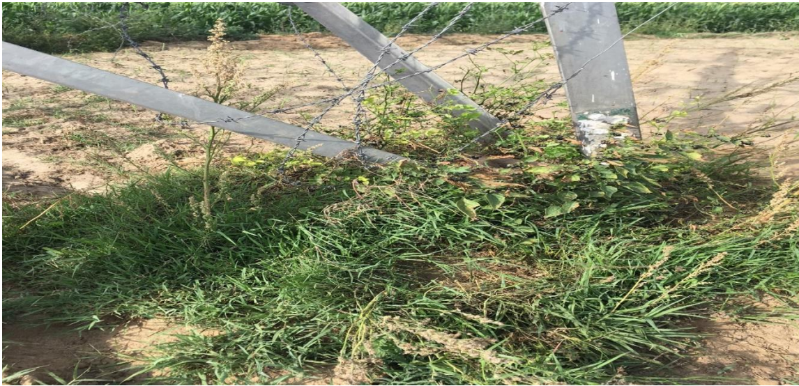
Figure 3. Damaged Anti Climbing Device (ACD)
