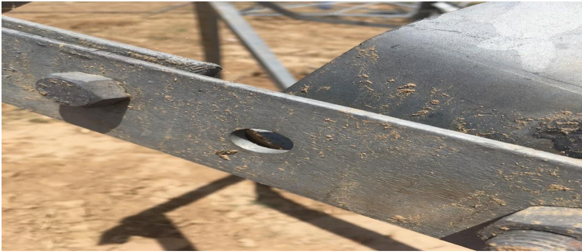
Figure 1. Missing bolt in bracing
