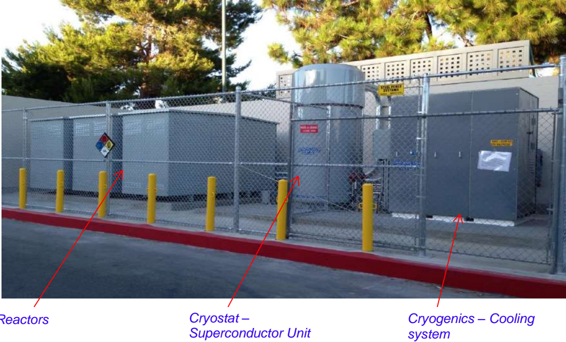
Figure 4 Silicon Valley Power, Santa Clara, California
