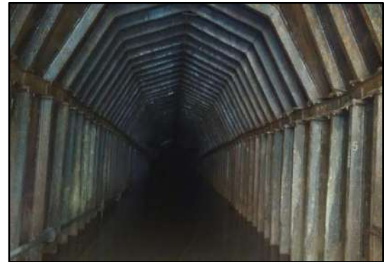
Fig. 8: Completely collapsed face of Adit-I
