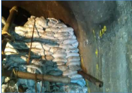
Fig. 7: Completely collapsed Face-IV of DT
