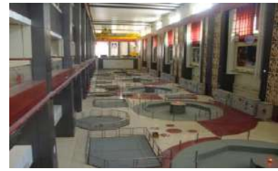
Surface Power House RHPS 412 MW
