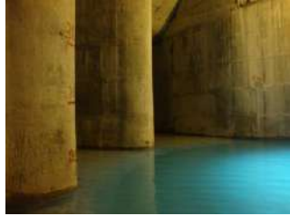
Pressure shaft bifurcations seen from pressure shaft 3
