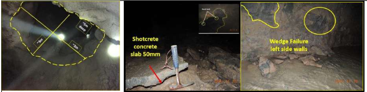
Figure-3 Cavity formation, damaged shotcrete & wedge failure due to presence of swelling clay
