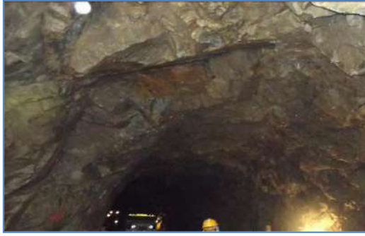
Fig. 5: Over break due to failure of wedges
