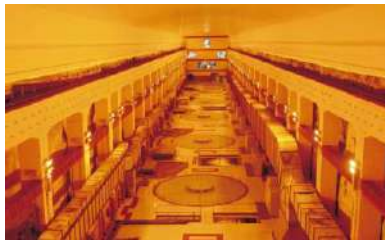
Underground Power House NJHPS 1500 MW
