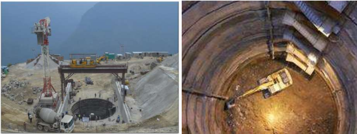
Figure 3: (a): Panoramic view of Surge shaft showing installed cranes. (b) Excavation being carried out by excavator (mechanical means).
