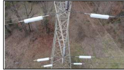
Fig2: PFC installed on Transmission line, Source: Ref [1]
