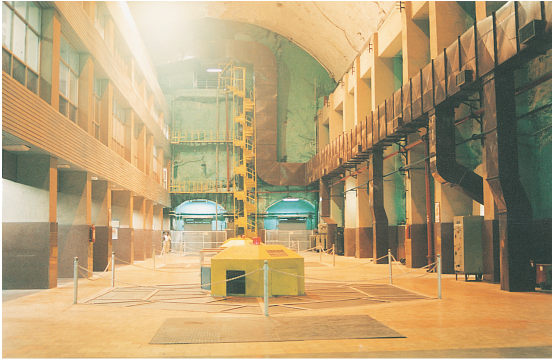
Machine Hall of Bhabha Power House 3x40 MW
