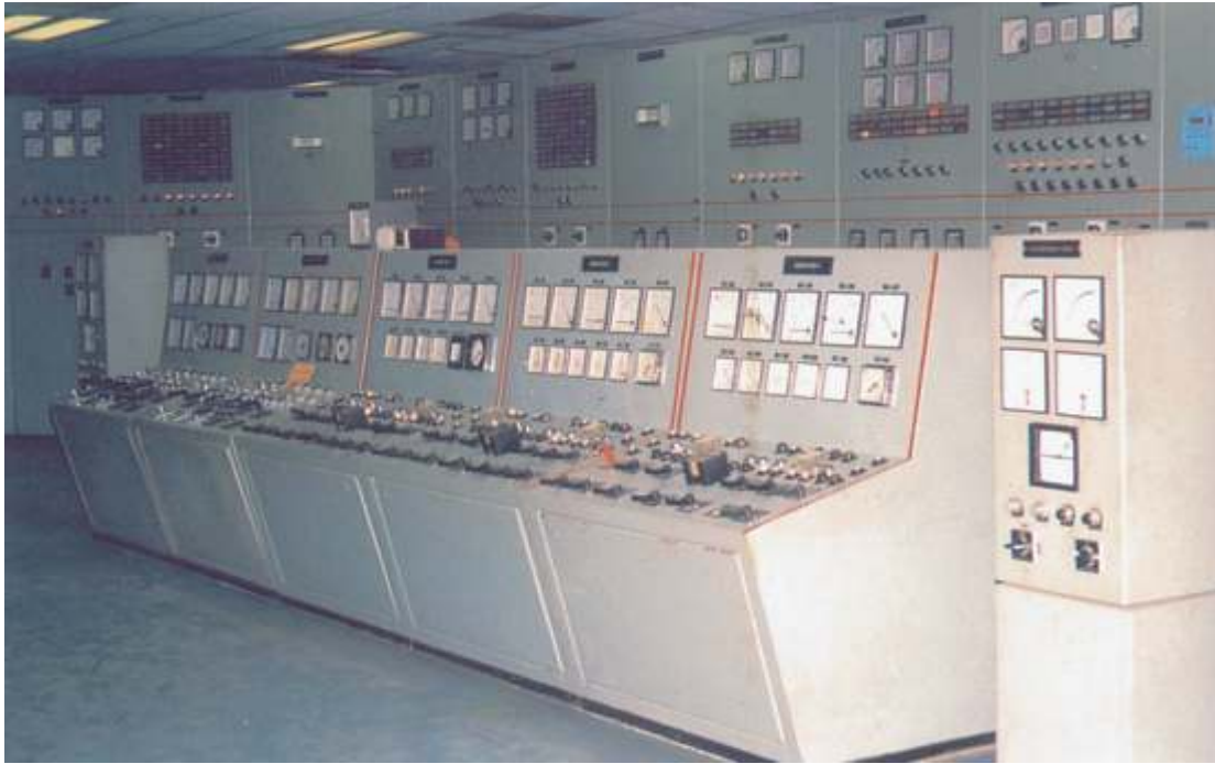
Control Room, Rengali HEP
