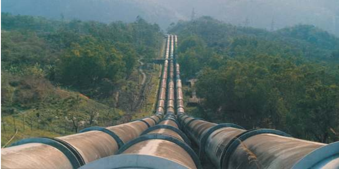
105 MW Loktak Power Station (Manipur) - Penstocks
