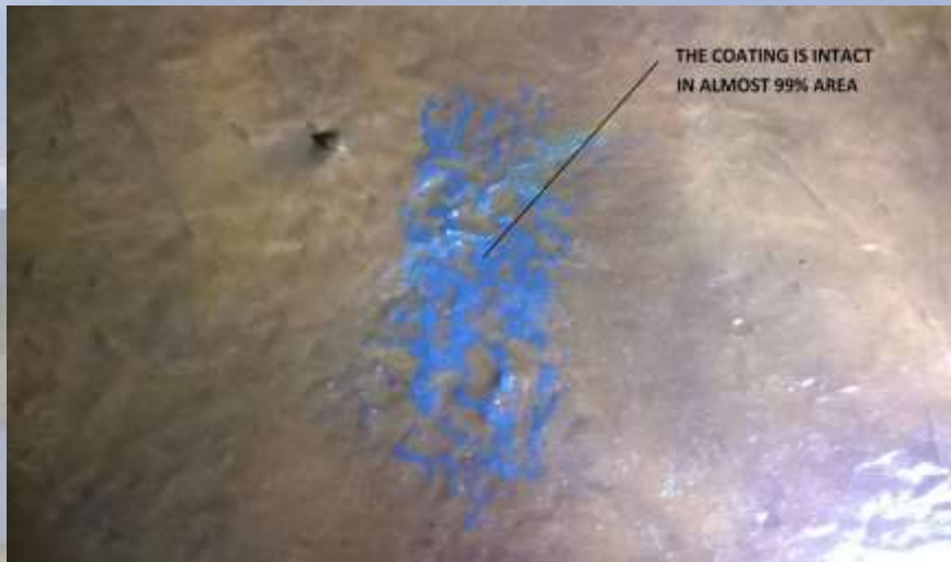
INSPECTION OF SPIRAL AFTER ONE YEAR OF APPLICATION OF LOCTITE COATING
