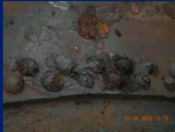
Severe corrosion on rivets
