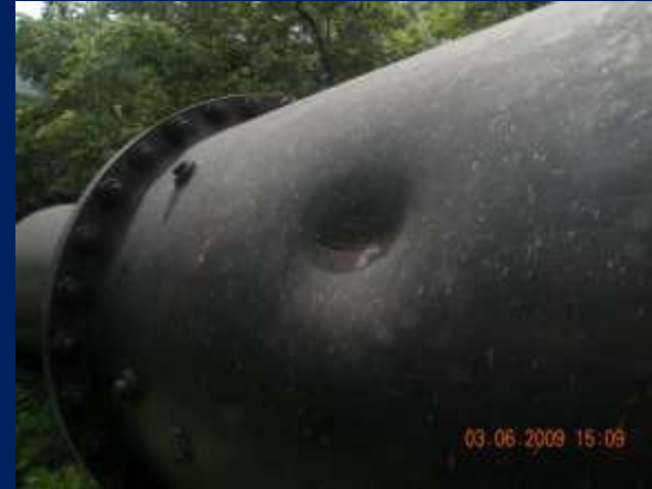
Severe dent on Penstock No. 1
