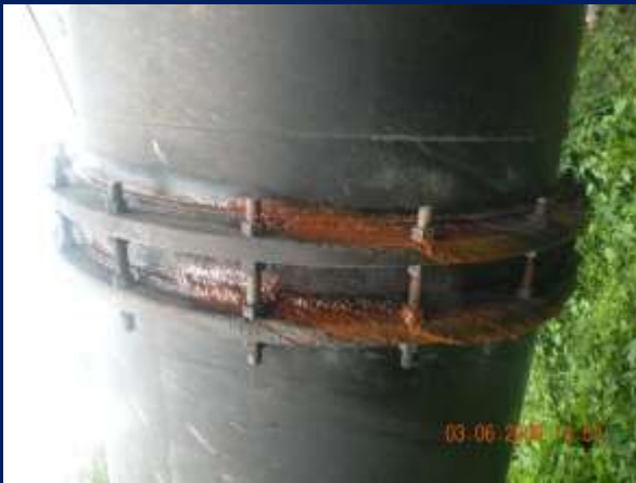
Flange leakage in Penstock No.4
