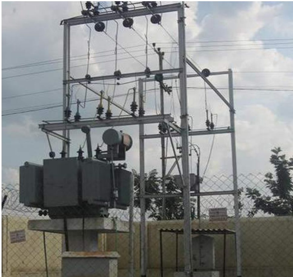
Plinth Mounted Distribution Transformer Sub-stations
