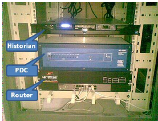
Fig 2. 3: PDC and other Equipments at NRLDC
