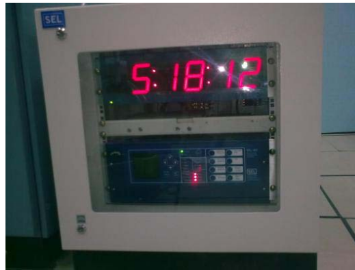
Fig 2. 4: PMU and GPS at Substation
