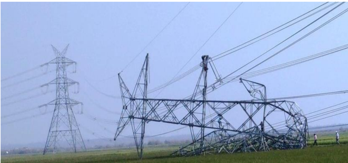
Tower at location no 15/1
