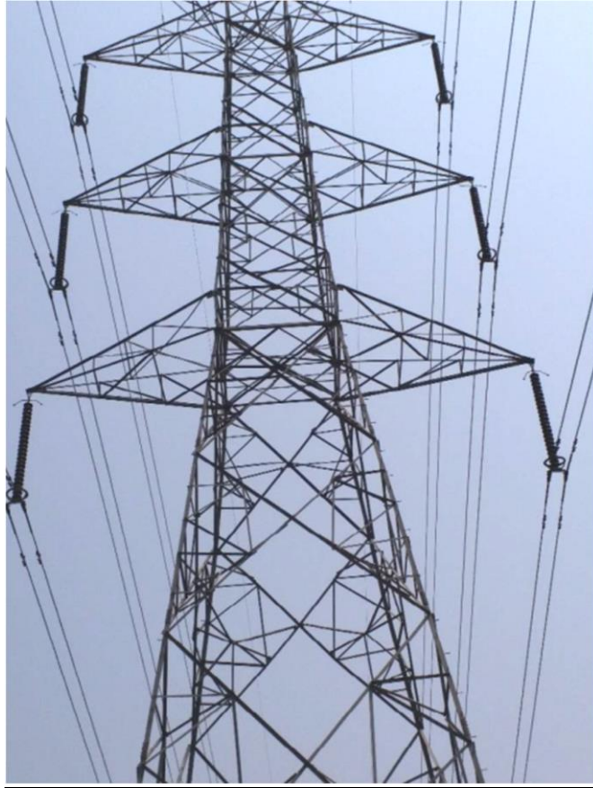
Tower at Loc. No. 407(DA+0)
