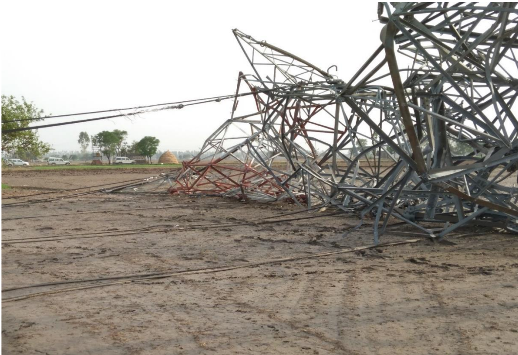
Tower at location no 59
