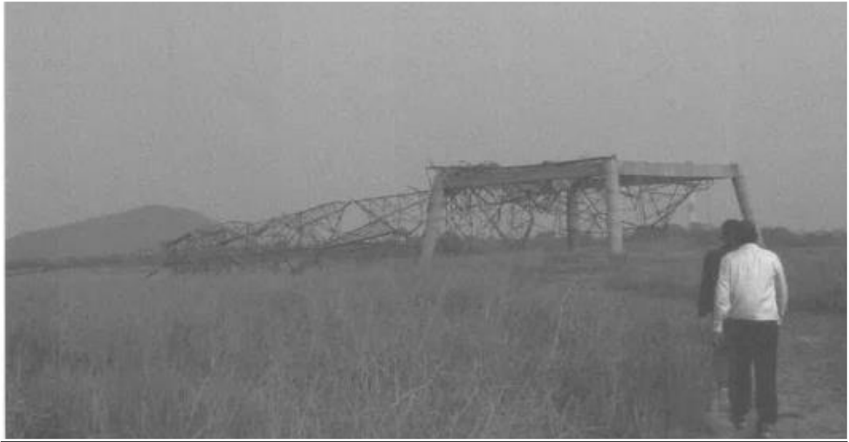
Probable Cause of Tower at Loc. No. 64
