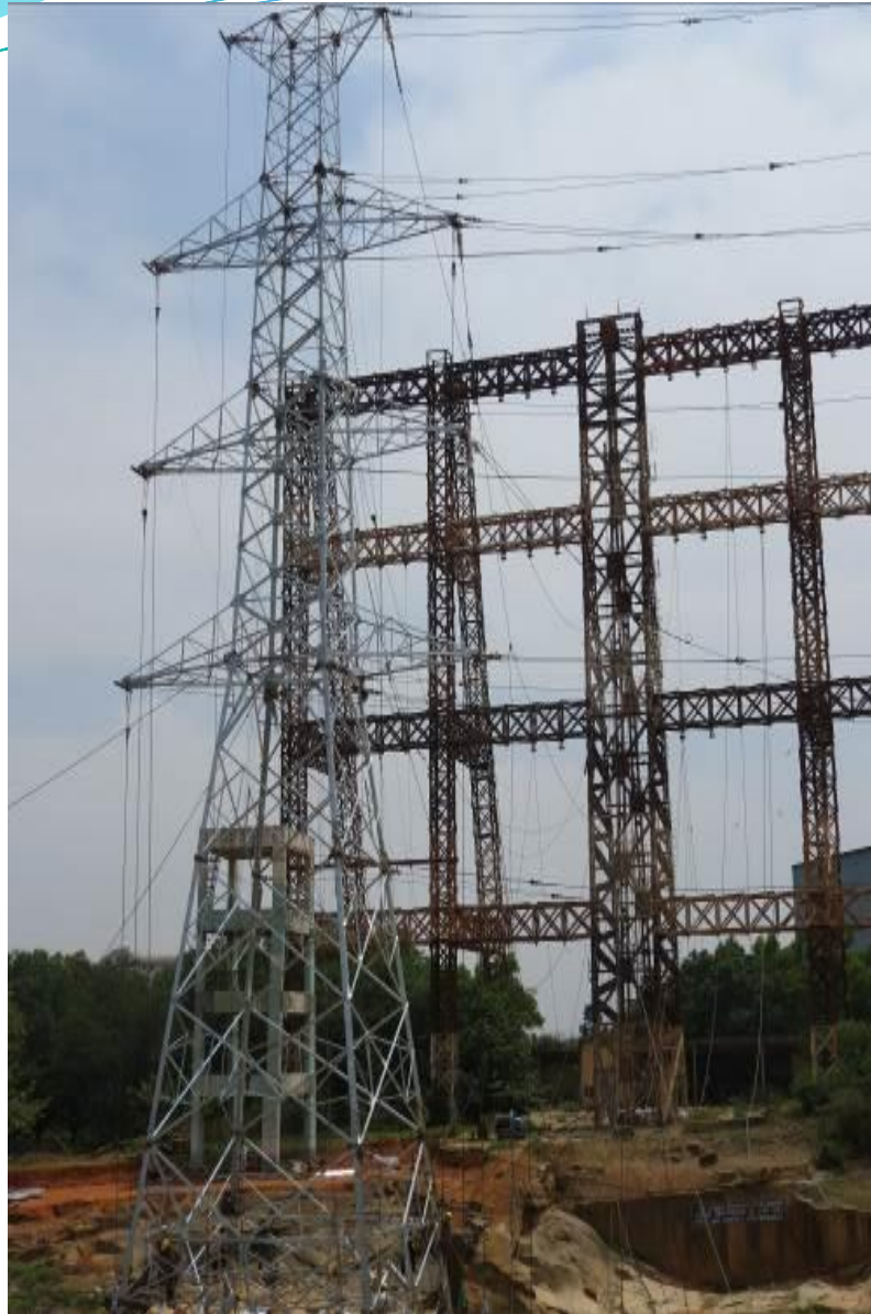
220 kV D/C Tension tower
