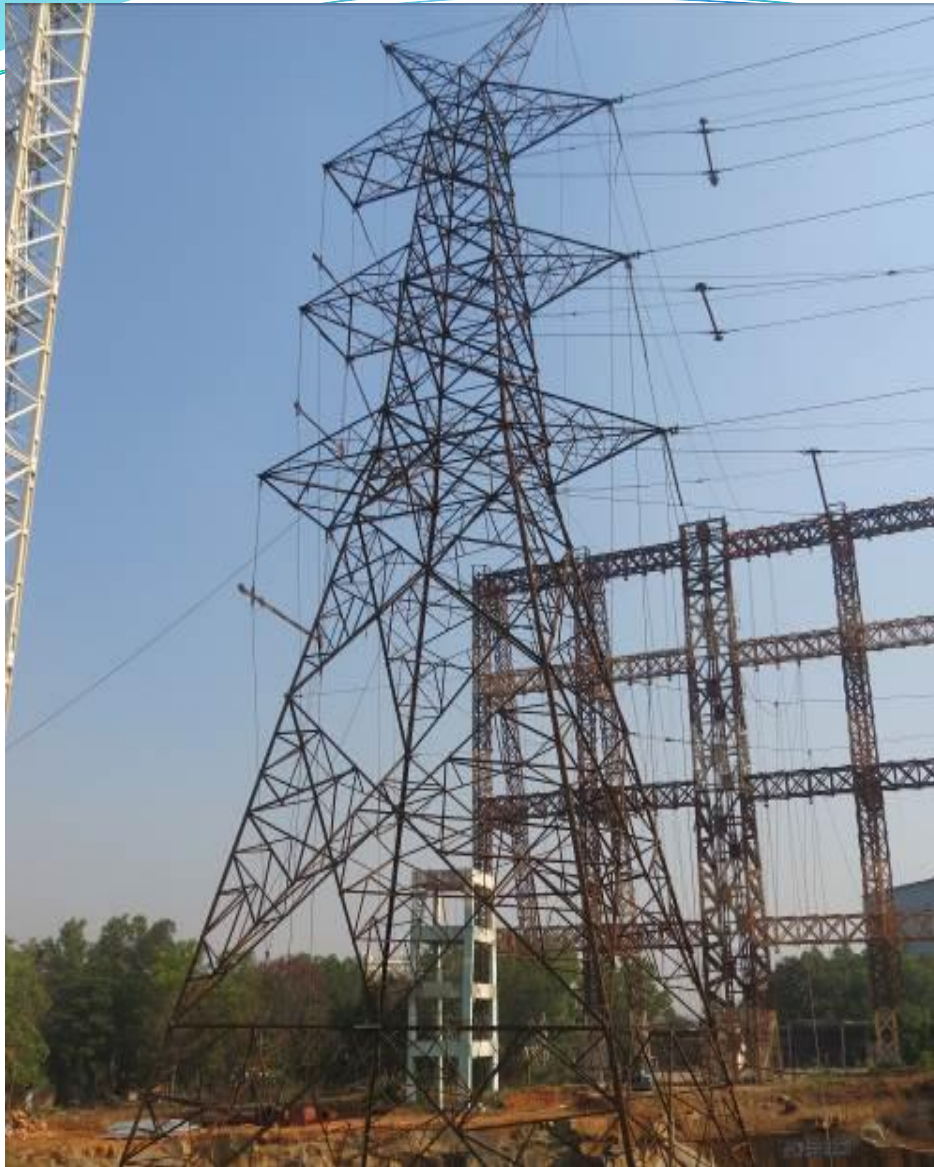
400 kV D/C Tension tower
