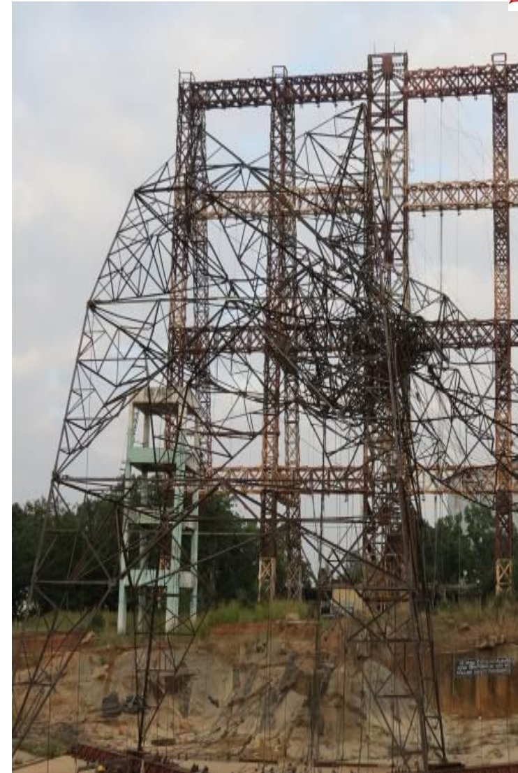
Failed during 95 % to 100 %
