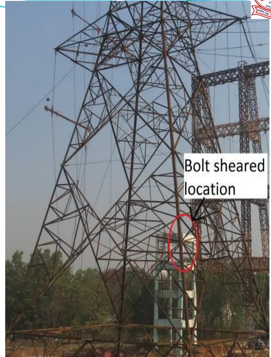
Failed at 95 % loads
