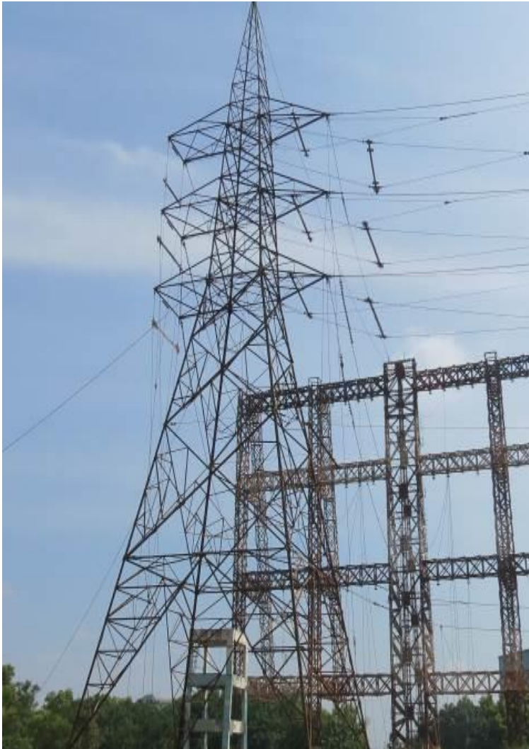
220 kV D/C Tension tower
