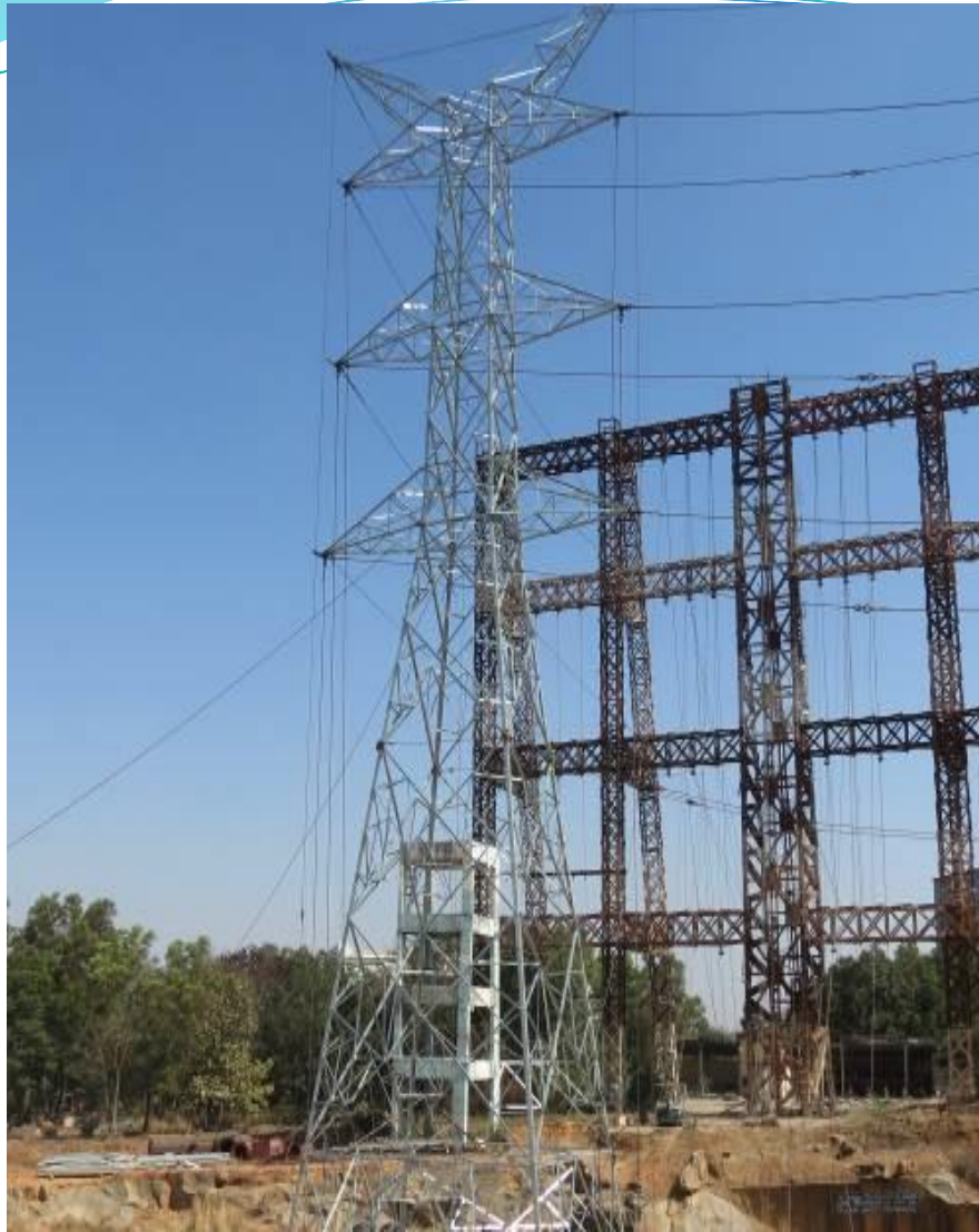
330 kV D/C Tension tower
