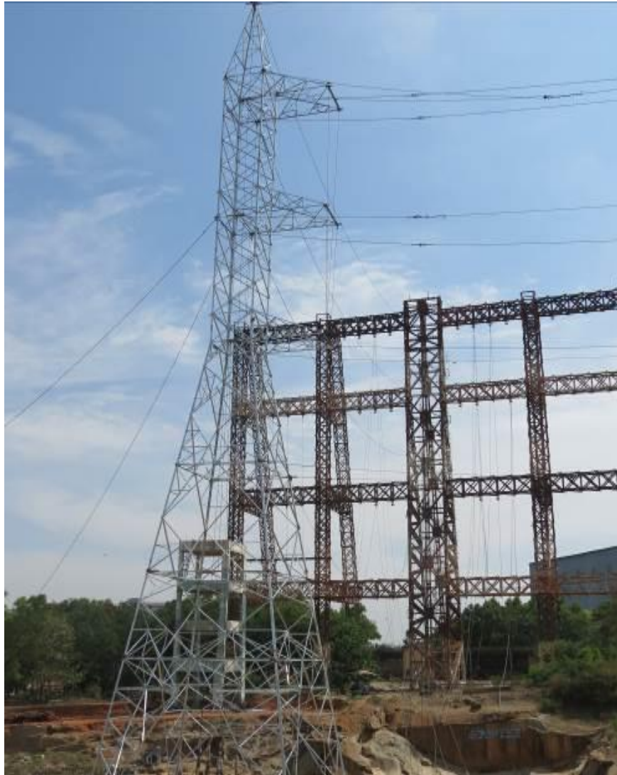
220 kV D/C Tension tower
