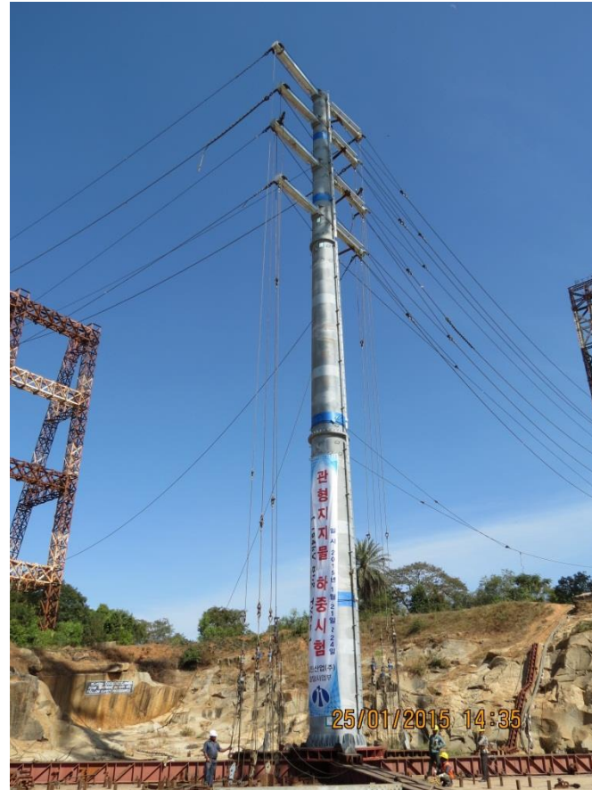
154 kV D/C Steel pole Korea
