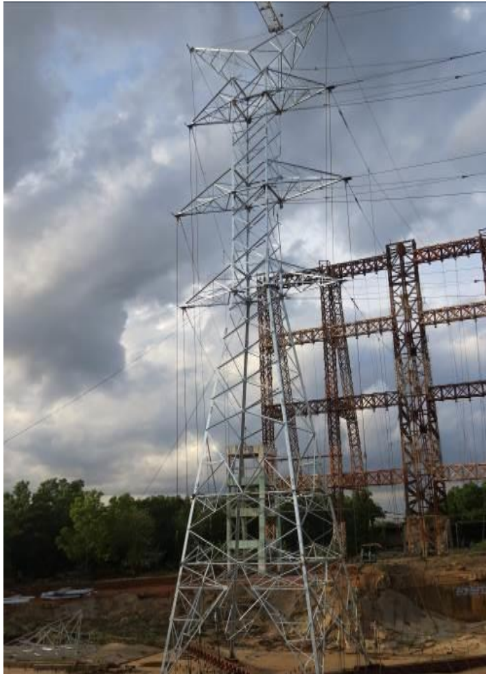
220 kV D/C Tension tower
