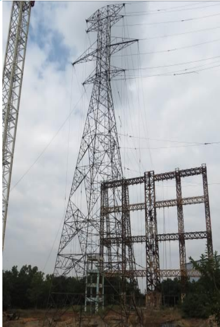
230 kV D/C Tension tower
