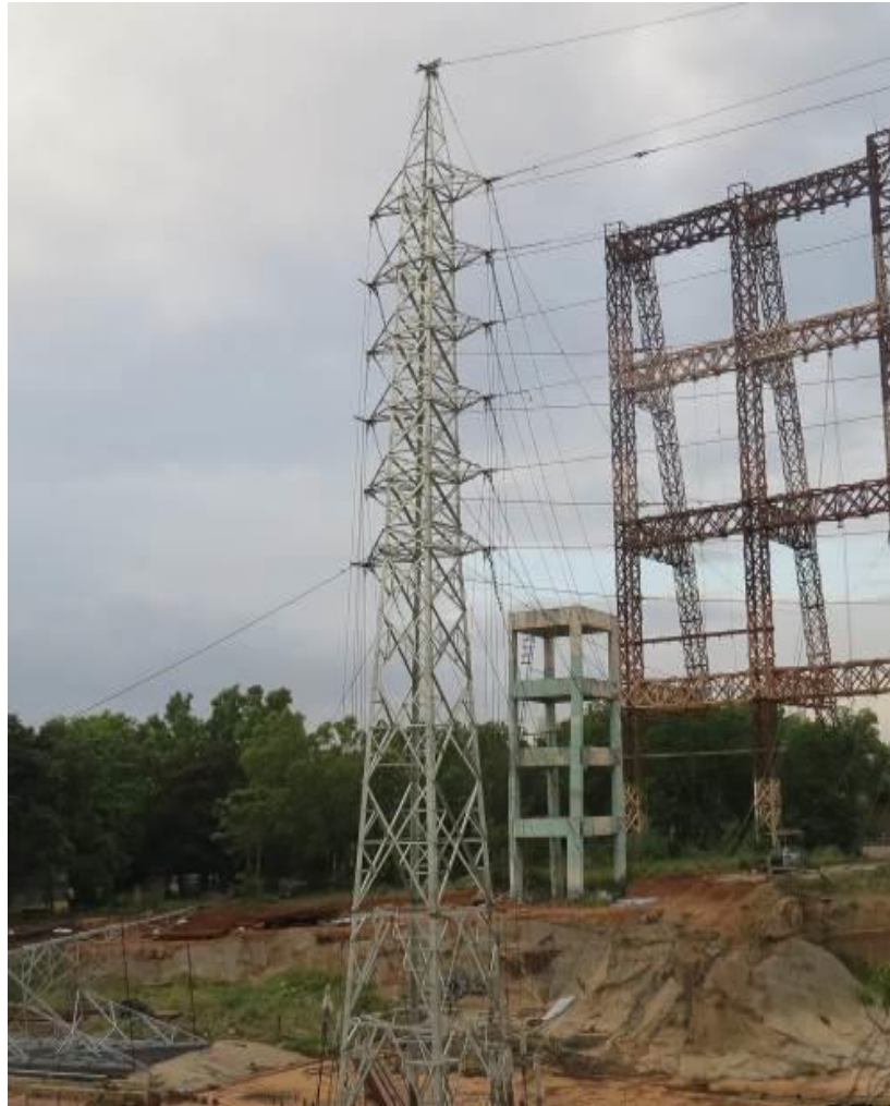
66 kV M/C Tension tower
