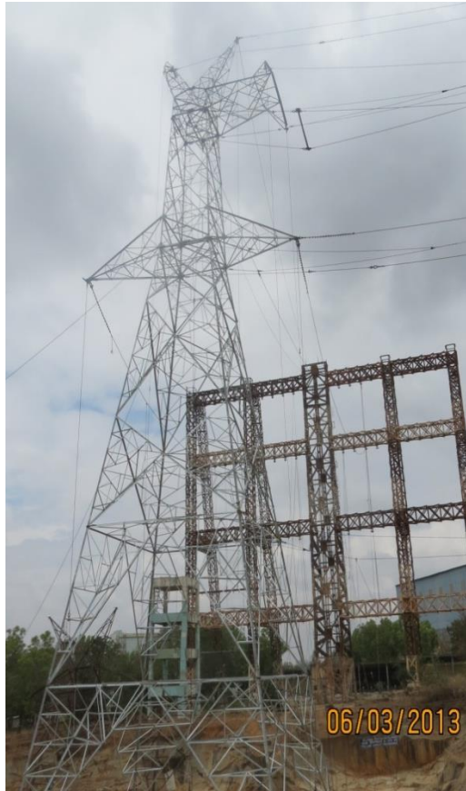
765 kV S/C Power Grid
