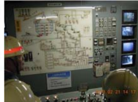
Control panel (KCM)
