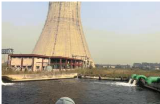
Condenser cooling water and cooling tower
