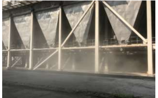
Hopper at the bottom of the electric dust collector
