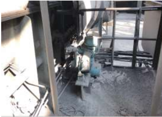
Forced draft fan control drive collector
