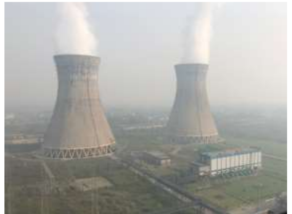
Condenser cooling towers
