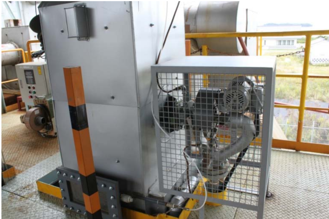
Figure 3.4-3 Appearance of soot blower
