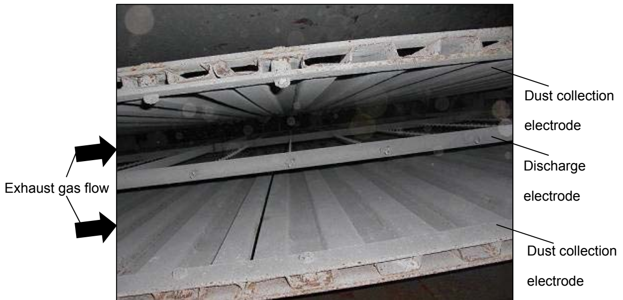
Figure 3.2-2 Inside of the dust collection chamber
