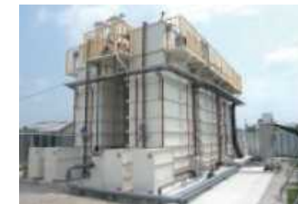
Pilot Plant for Low Energy Consumption Tech. by MBR (Membrane Bioreactor)
