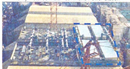
Newly Installed MEEP at Rihand Power Station
