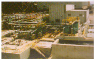
General wastewater treatment plant
