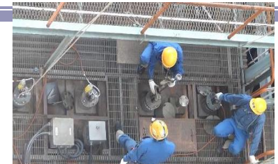
Leak Ammonia at SCR System
