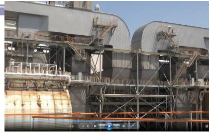
Inlet & Outlet Duct
