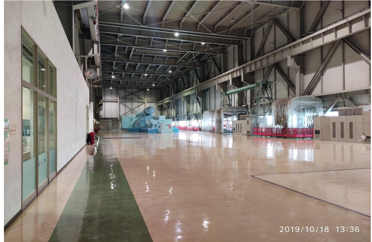
Reihoku: Turbine Floor
