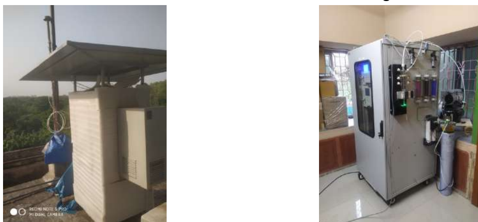
Figure 2.7: Left-side image is showing one of our standalone air-conditioned portable hut with SO 2 gas analyzer kept on the rooftop of a three-story building at one of the measurement site and the right-side image is of the same system kept inside a room in another measurement site.
