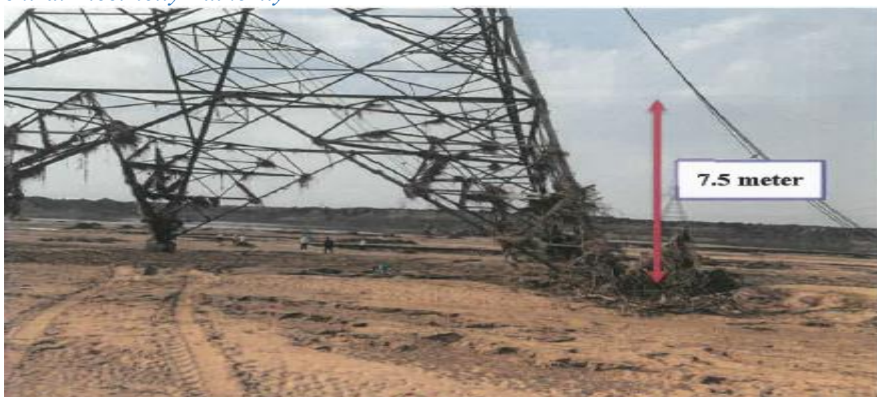
Fig 5(c). Tower at Location No.: 246 (D+0)-Debris Observed
