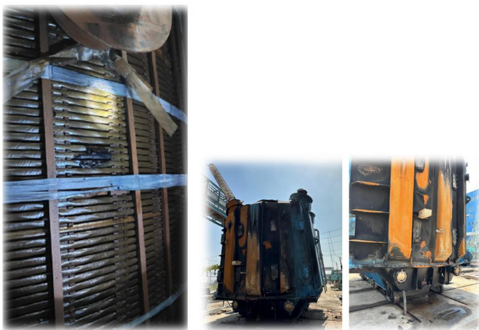
The Arching spot and burnt Transformer
