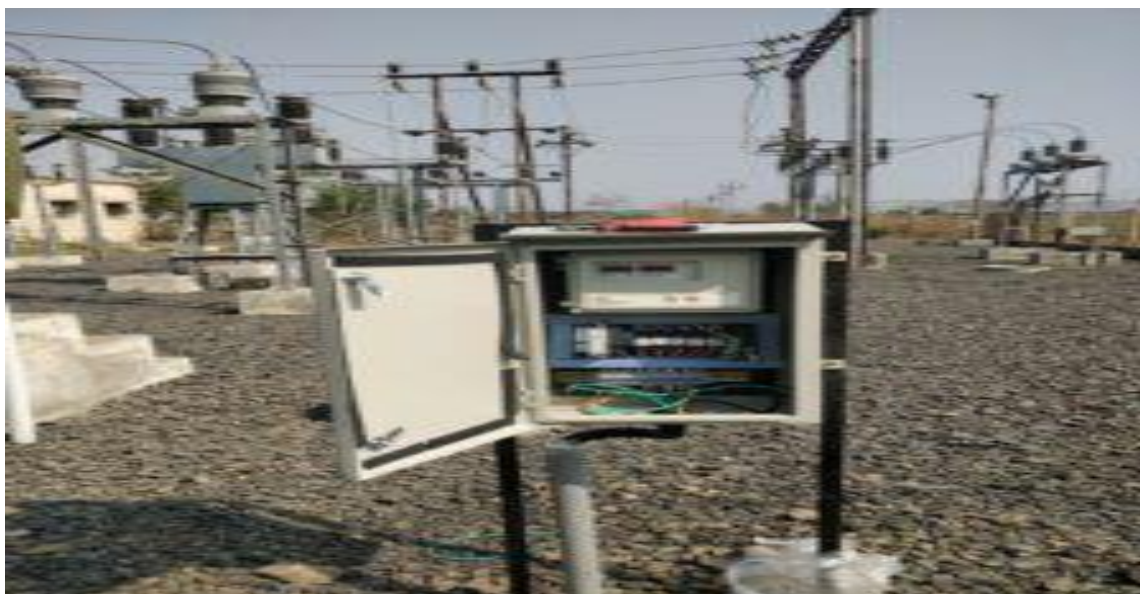
RT-DAS- Sub-station Monitoring
