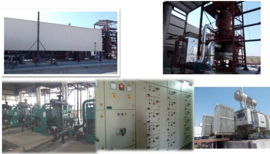
Figure 5-5: 1 MWe biomass gasifier installed in Mullana, Ambala, Haryana. [19]
