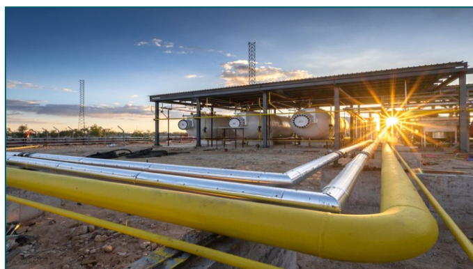
Figure 4-13. Integrated green hydrogen and green ammonia plant, Bikaner, Rajasthan. [22]
