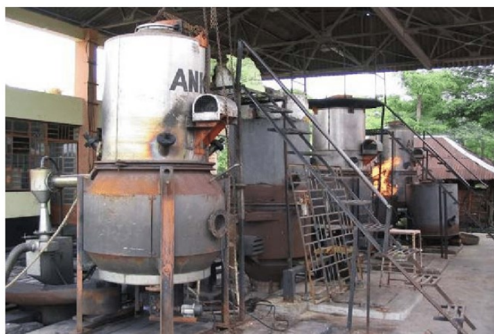
Figure 5-4: 5 x 100 kW biomass gasifier at Gosaba Island, West Bengal, India. [17]
