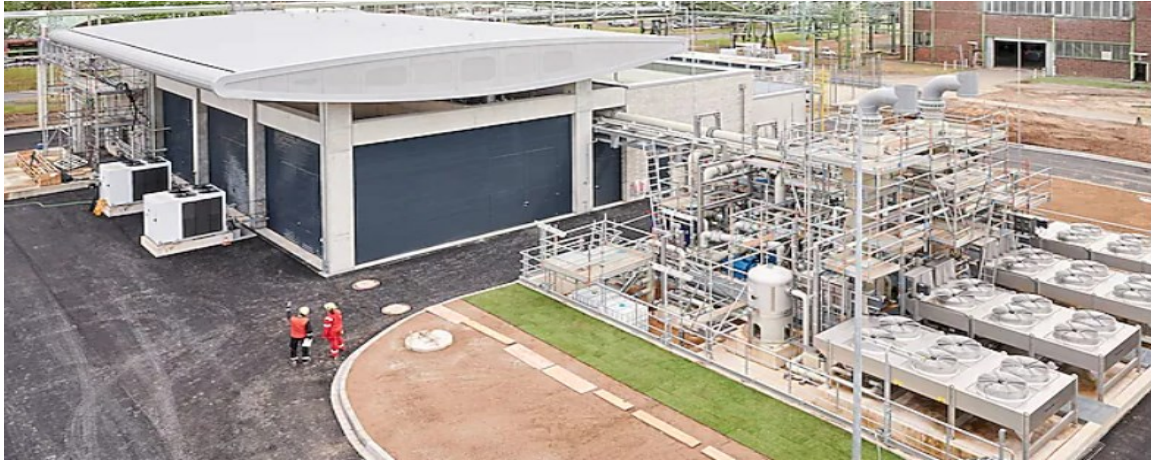
Figure 2-10: MW PEM electrolyser at Shell's Rhineland Refinery in Wesseling.
