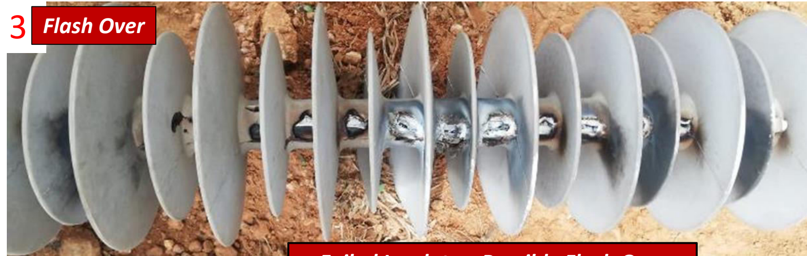
Failed Insulator: Possibly Flash Over
