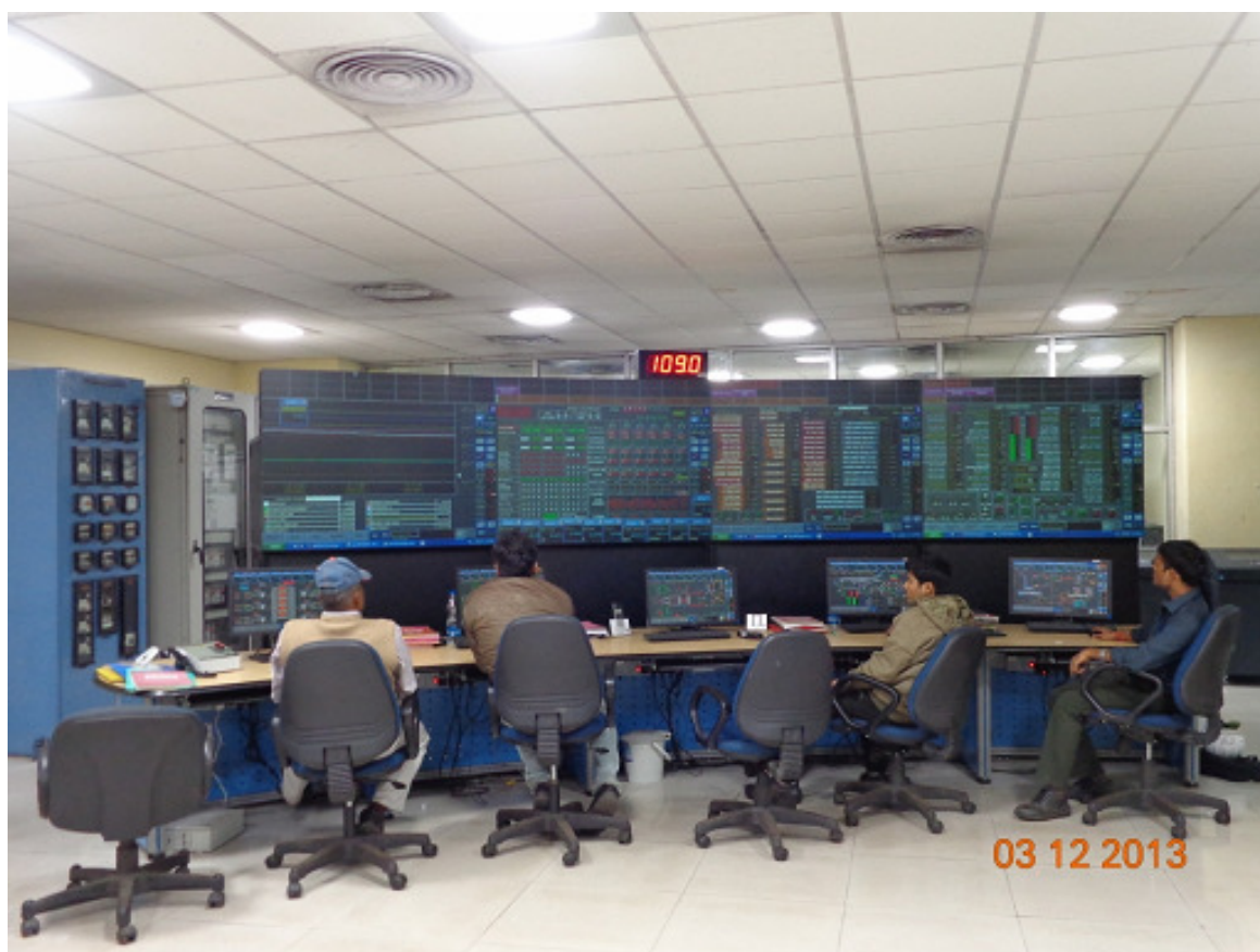
Control room of Muzaffarpur TPS after Renovation
