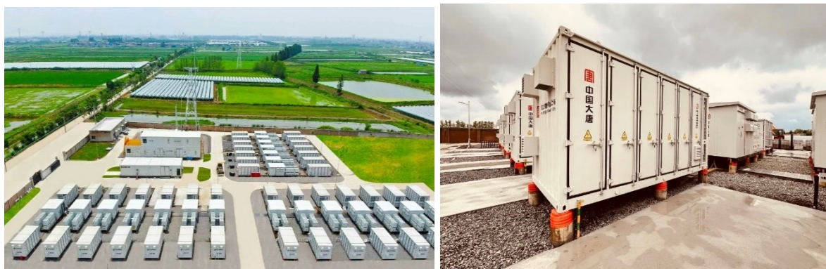
Figure 3-2: 100 MW/200 MWh Sodium-ion energy storage station Datang Hubei China [29].
