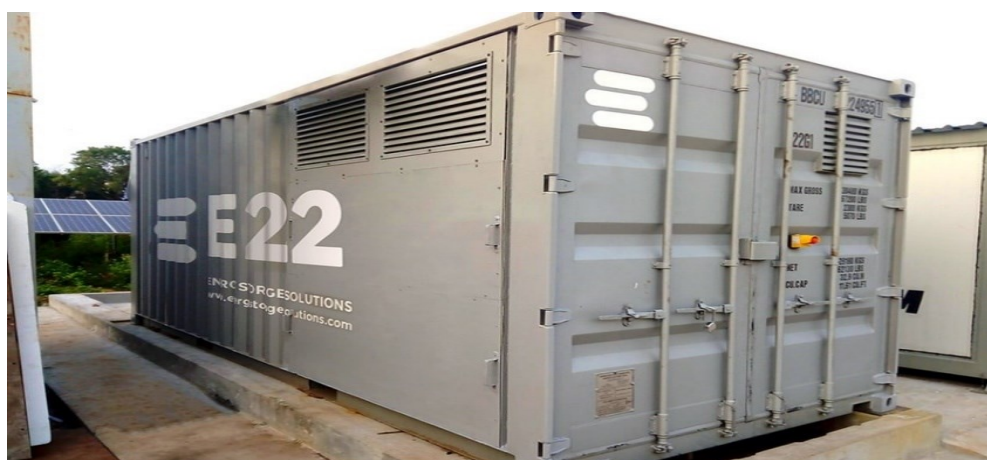
Figure 5-3: BHEL 50 KW VRF plant battery [30].
