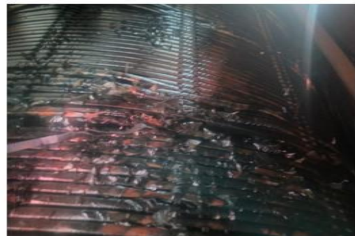
Hv winding discs were found severely burnt
