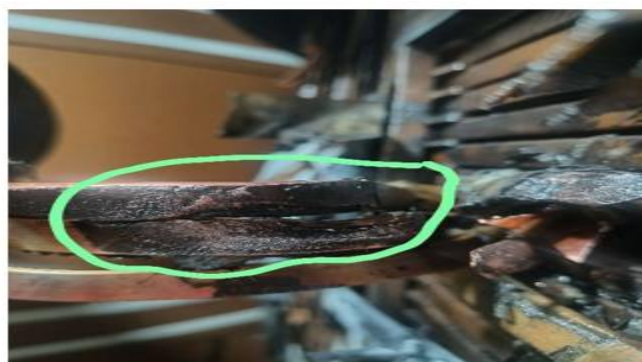
2 No's of winding conductors were melted
