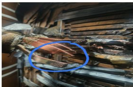
3nos conductor was found broken.
