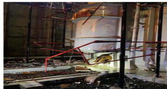
HV side inspection cover got busted and found 2mtrs away from the reactor. Also, pressboard and paper insulation were came out.
