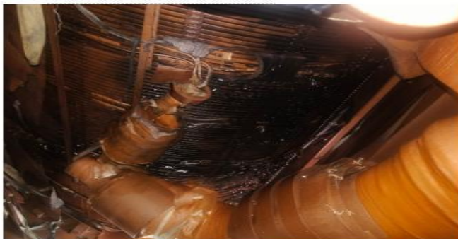
HV lead take out was found dislocated
