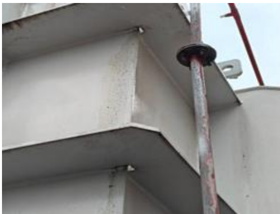
Cracks in HV side plate stiffeners welding side bottom near to B phase joints towards B Phase
