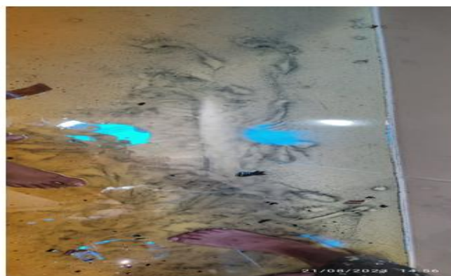
Carbon Powder on tank floor
