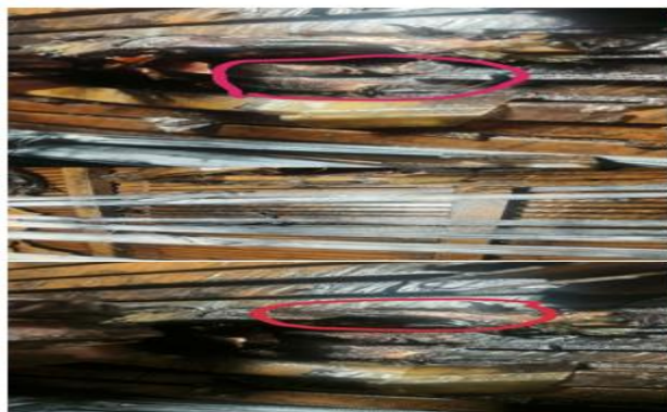
4No's disc layer conductor were found melted
