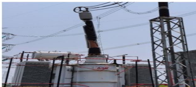
Physical damage of HV bushing
