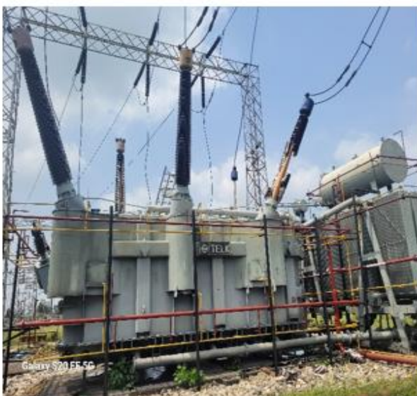
400kV B-Phase Bushing damaged
