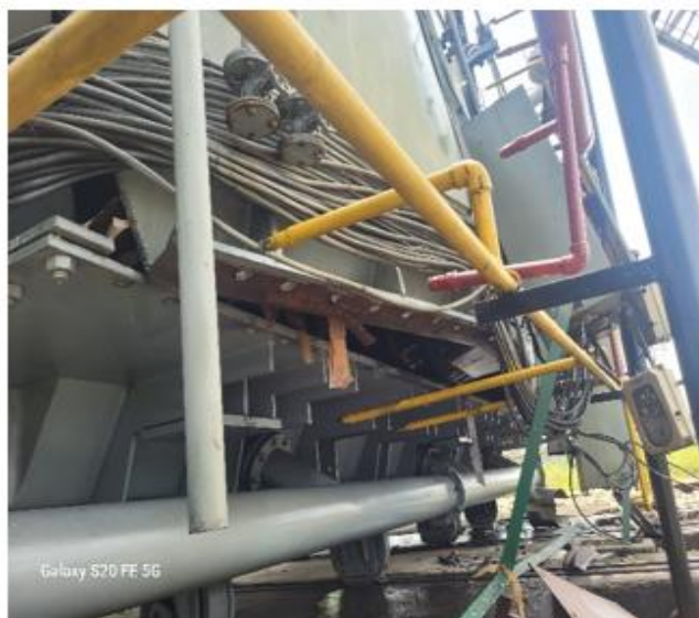
220kV Side main tank
