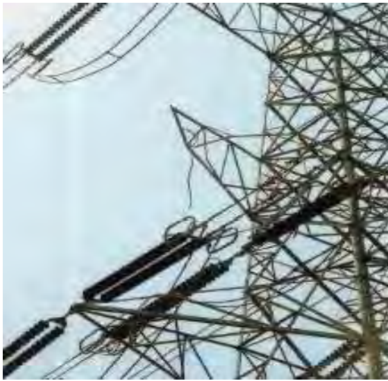
Tower loc. No. 159 (FD 30+3)
