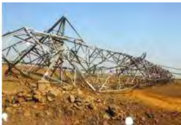
Tower loc. No. 165 (FD0)
