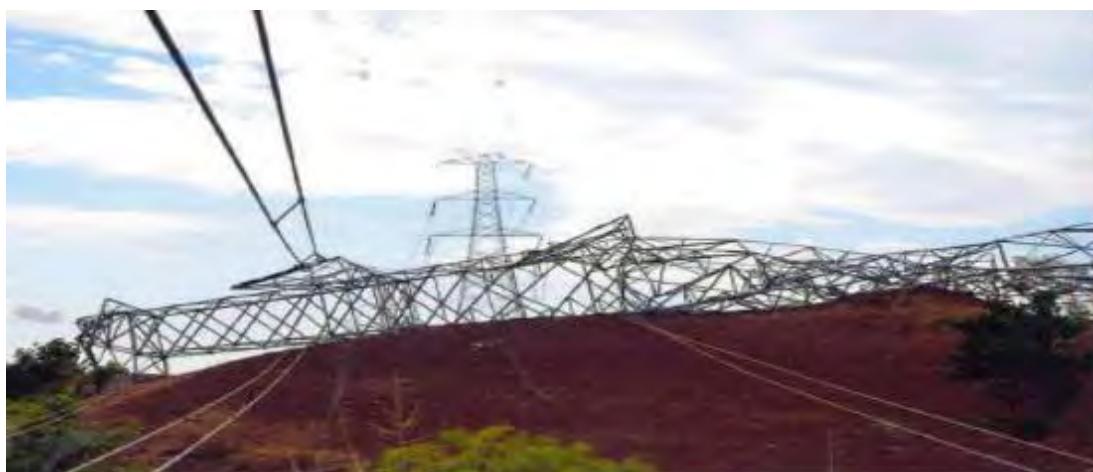
Tower at loc. No. 564
