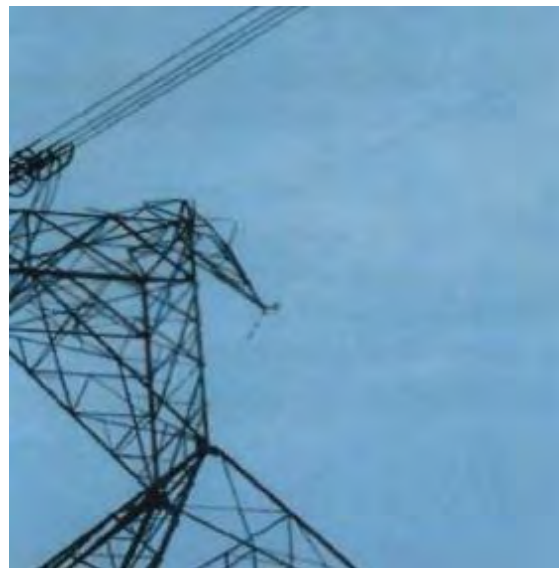
Tower at Loc. No.294 (C+25)
