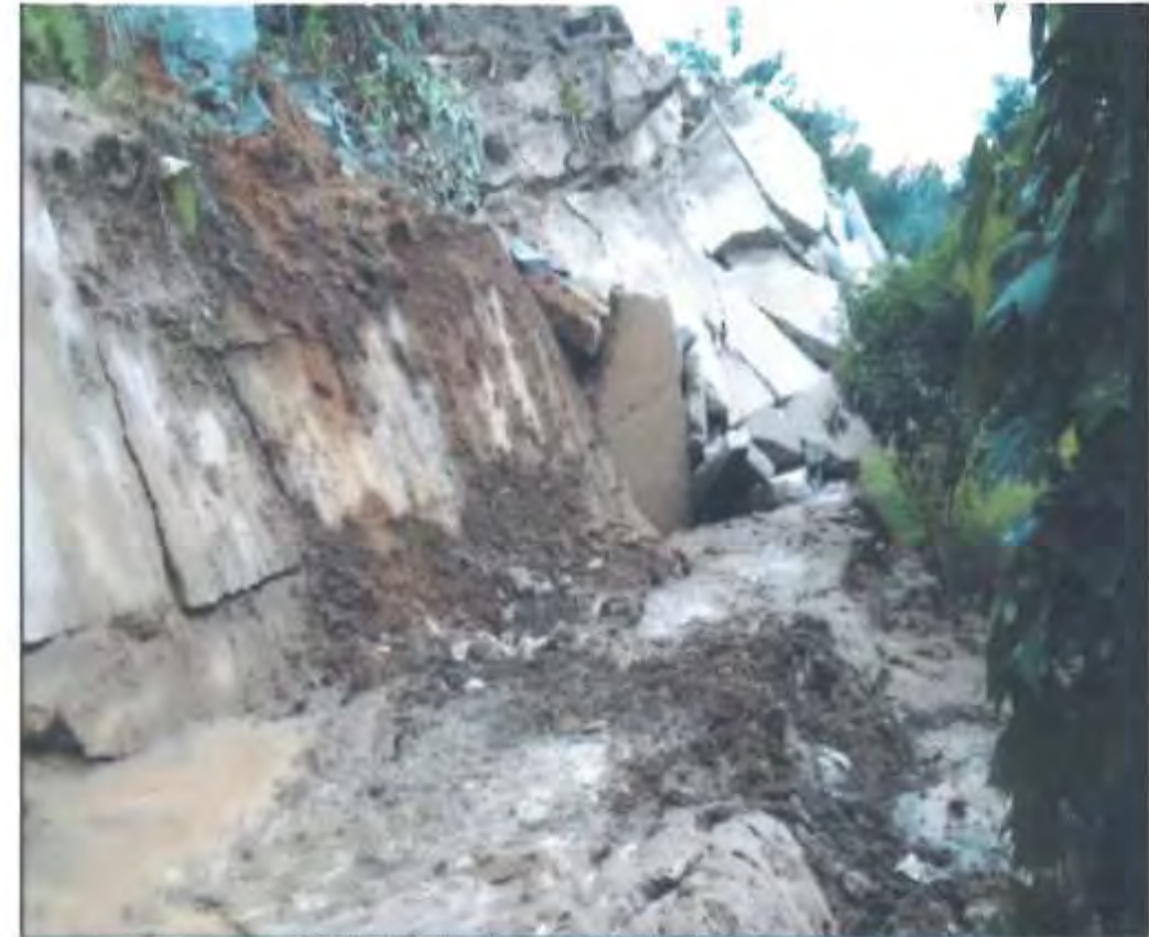
Destroyed NH-54 due to landslide (below tower location 377)
