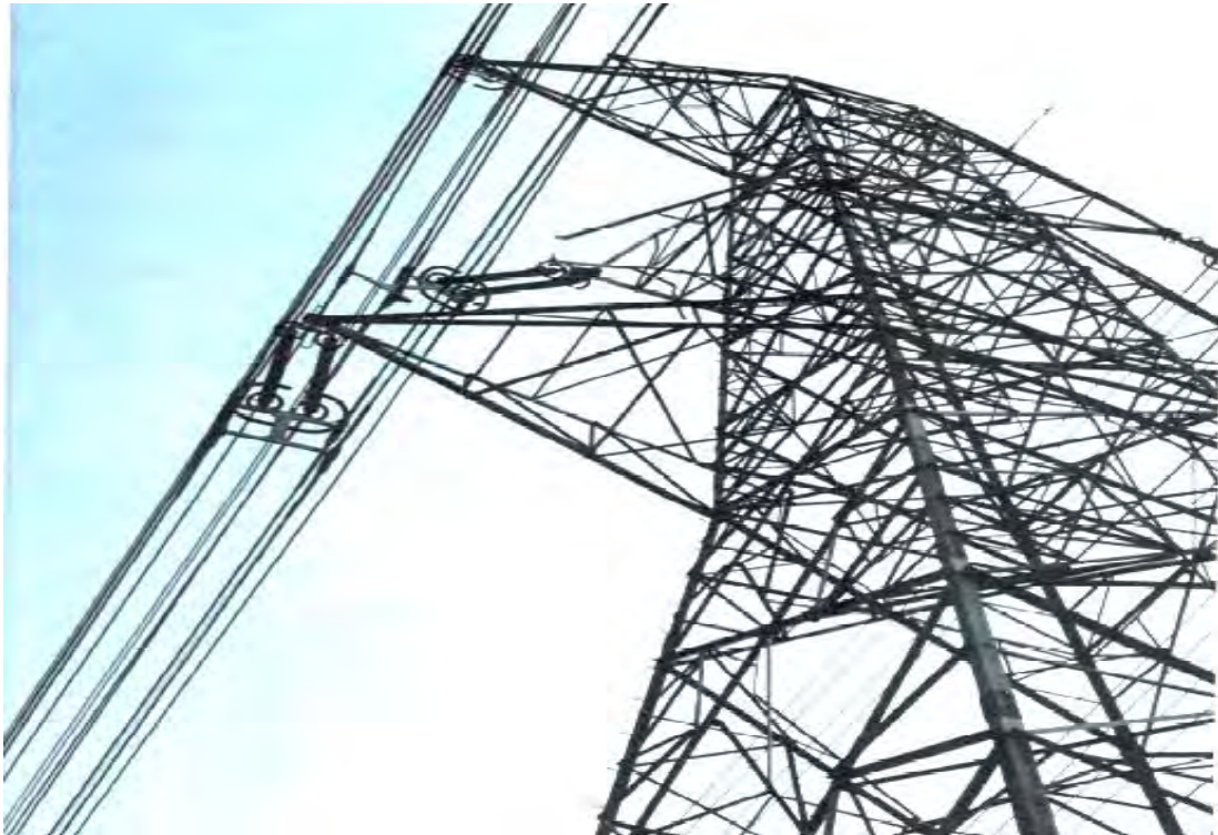
Tower at Loc. No.391 (DA+0)
