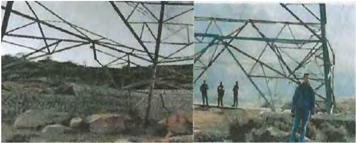
Bulging of Tower at Loc. No.144 (DB+0)
