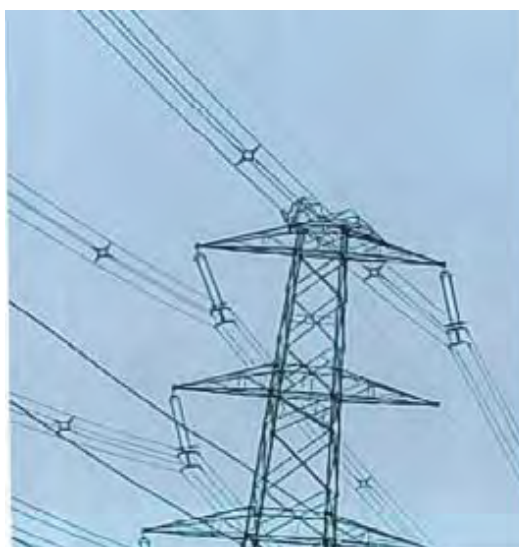
Tower at Loc. No.390 (DA+0)
