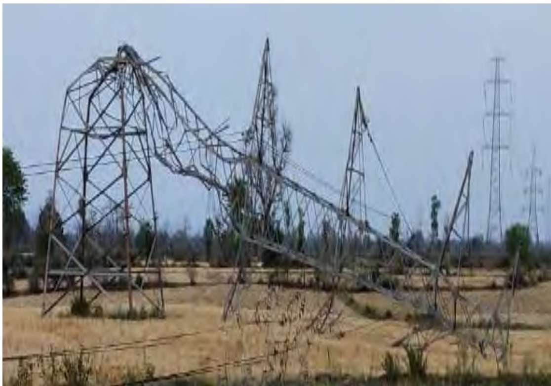
Tower Location No. 948 (DA+0)
