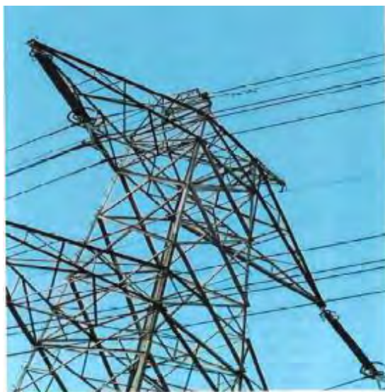
Tower at Loc. No.388 (DA+0)
