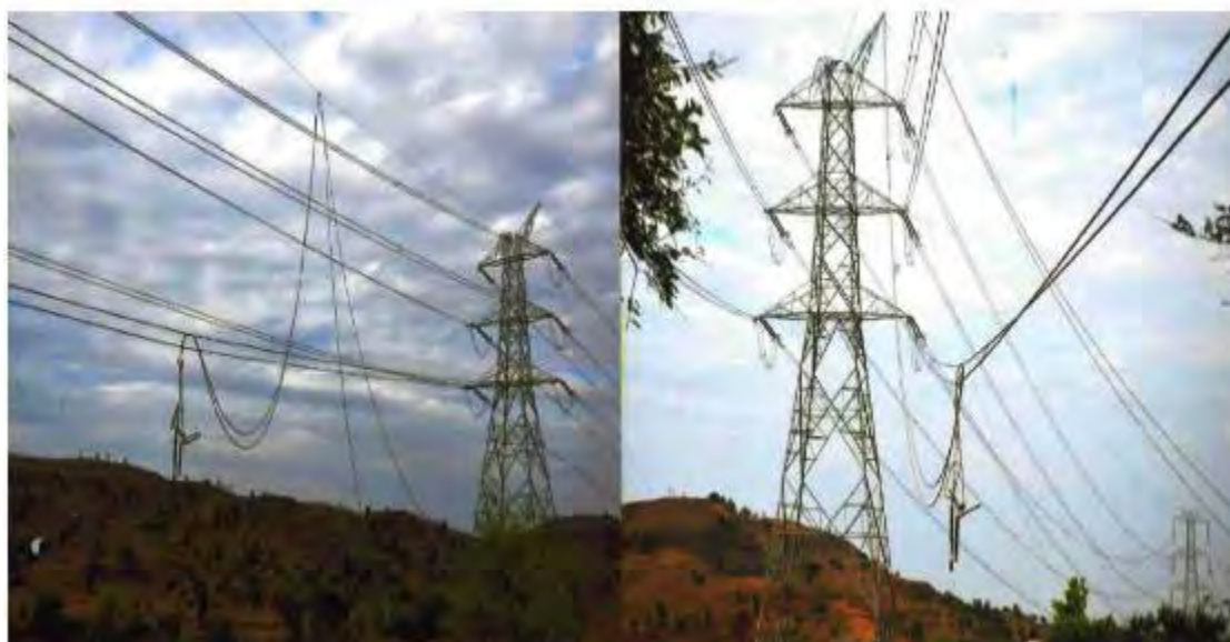
Tower at loc. No. 566
