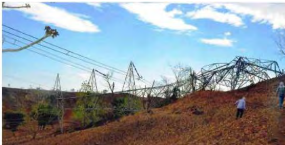
Tower at loc. No. 565
