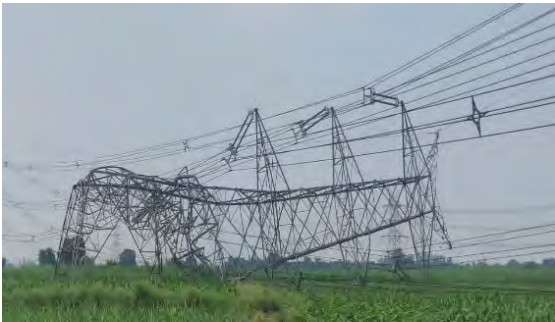
Tower at Loc. No.389 (DA+0)
