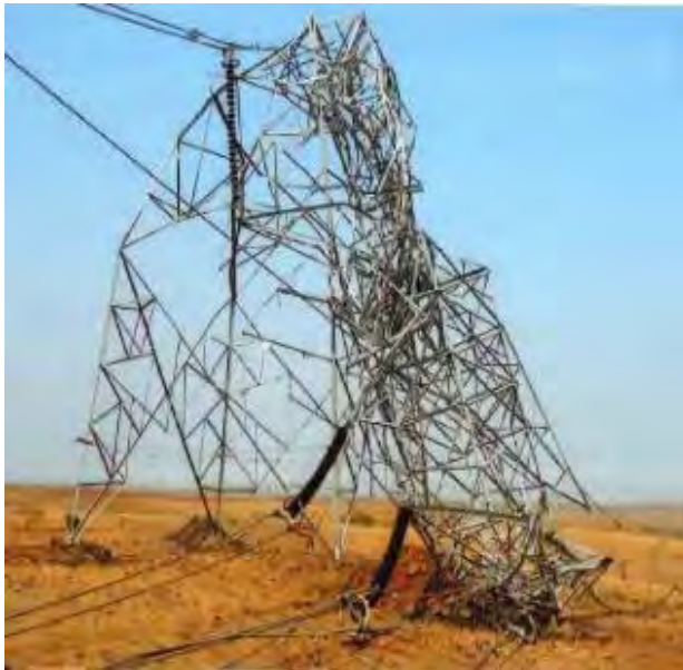
Tower loc. No. 161 (FD 0)
