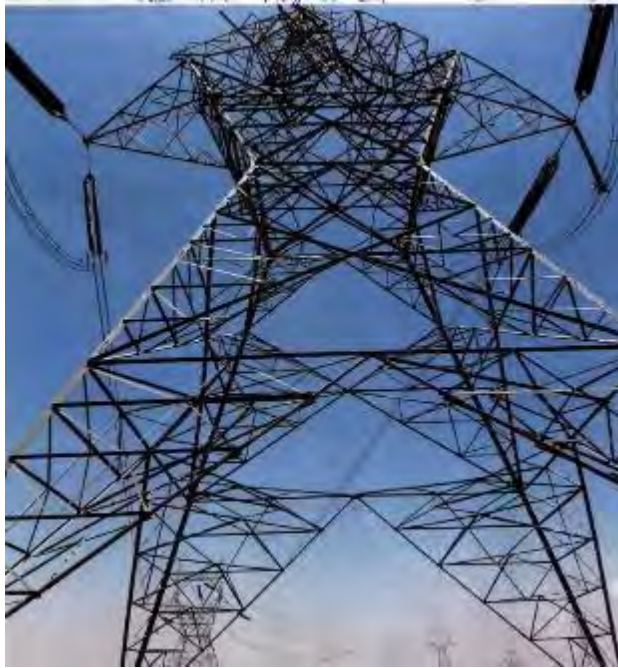
Tower at location No. 355 (61/0(TTC+3))
