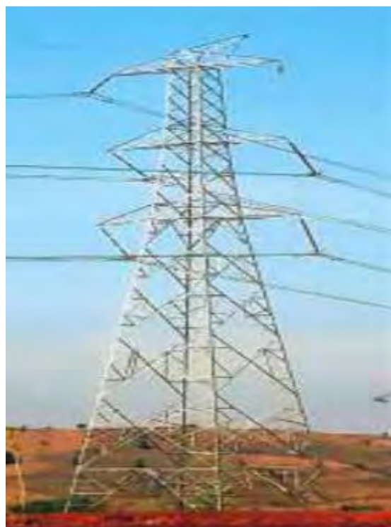
Tower at loc. No. 563
