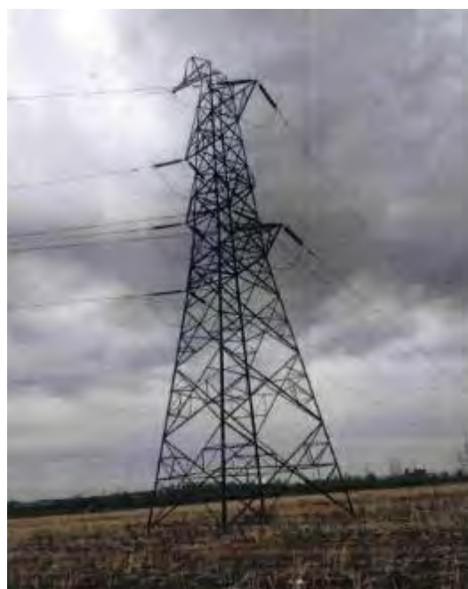
Tower at loc. No. 94
