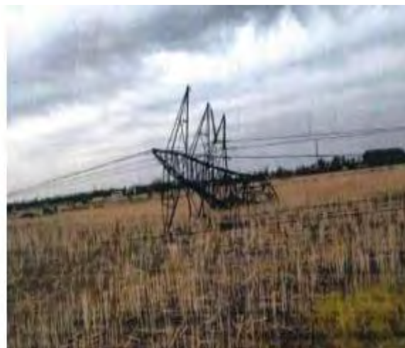
Tower at loc. No. 93
