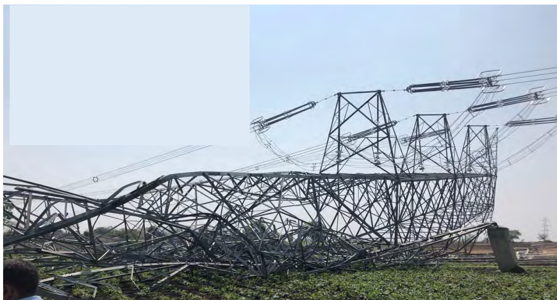
Tower at location No. 3/0 (DD+30+RC 3)
