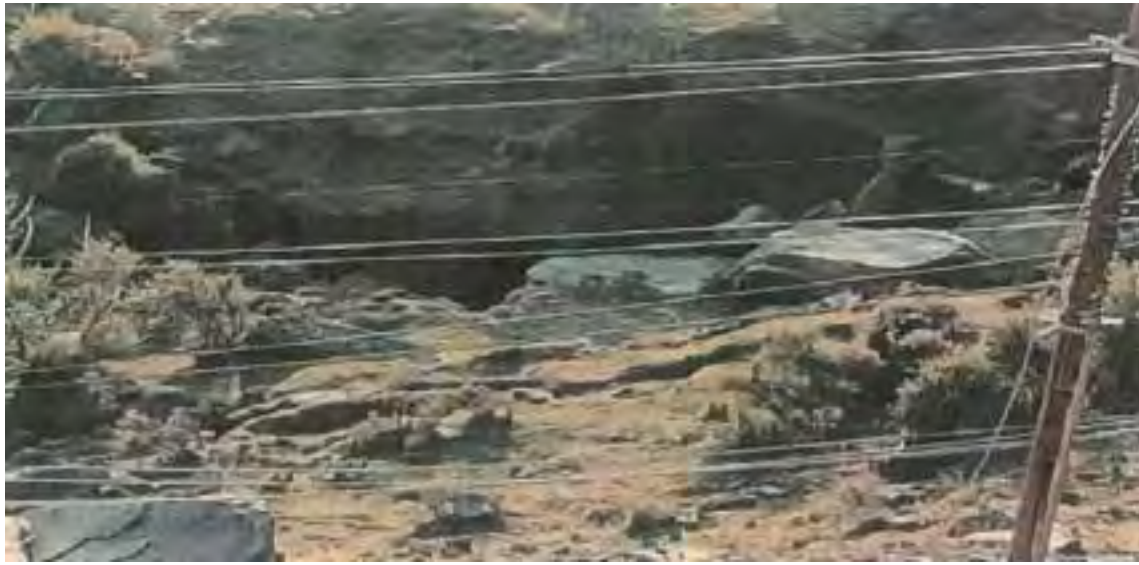
Cracks near Tower at location no. 144
