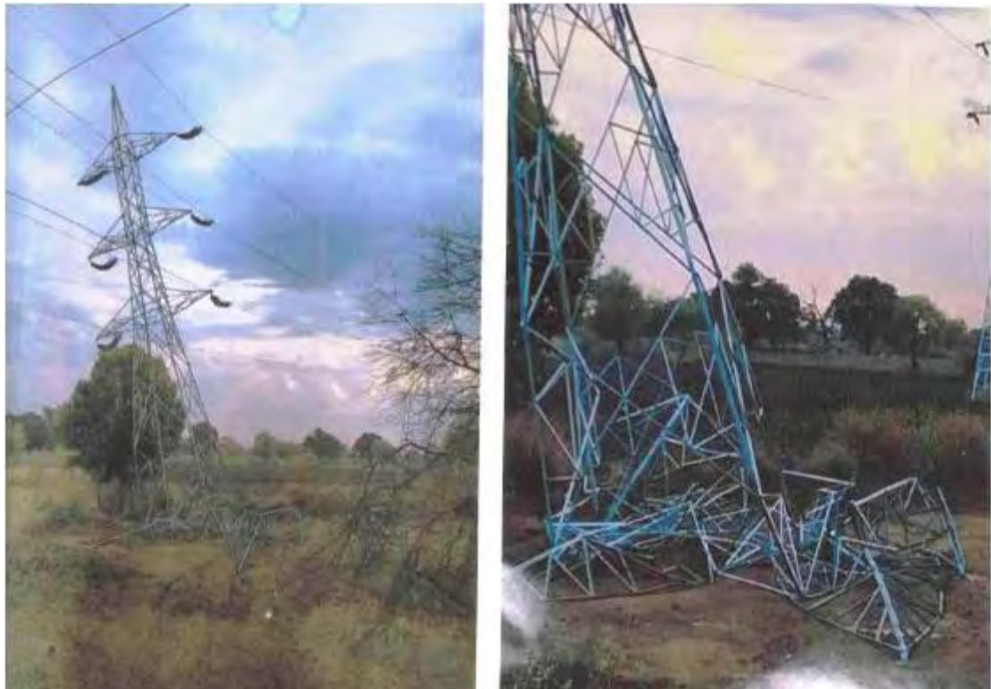
Tower at location No. 11A
