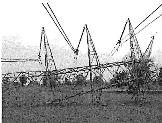
Tower at Loc. No.237 (DA+6)
