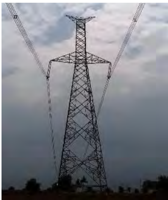
Tower at location No. 435 (A+3)
