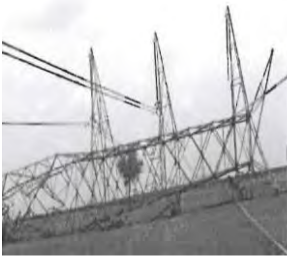
Tower at Loc. No. 239 (DA+3)
