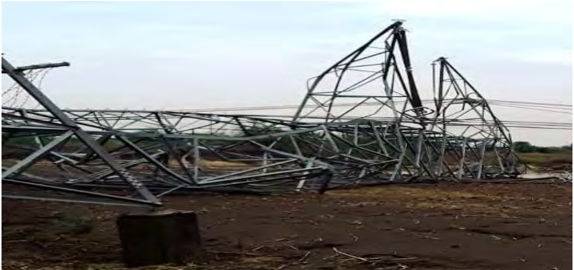
Tower at location No. 431 (A+3)
