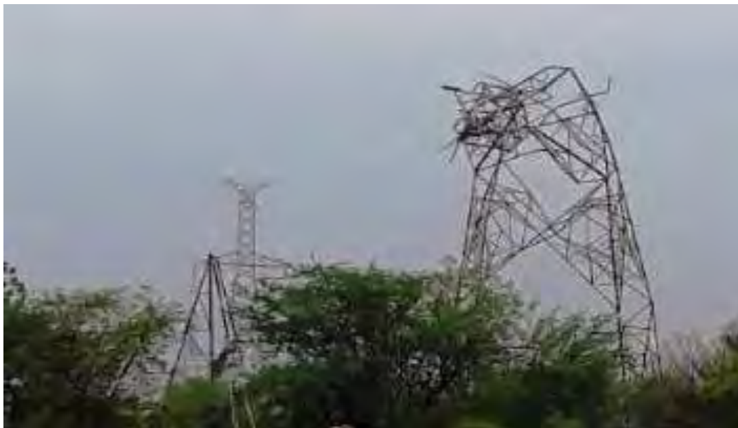
Tower at location No. 434 (A+0)
