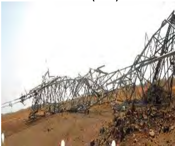
Tower loc. No. 163 (FD 0+3)
