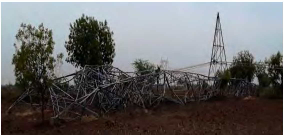
Tower at location No. 433 (A+0)
