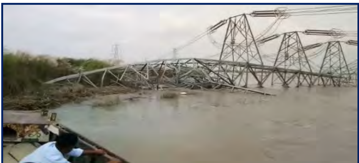
Tower at loc No. 26/0 of Barh-Motihari Line (after failure)
