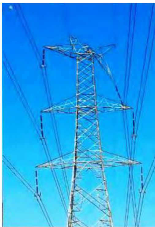
Tower at loc. No. 562
