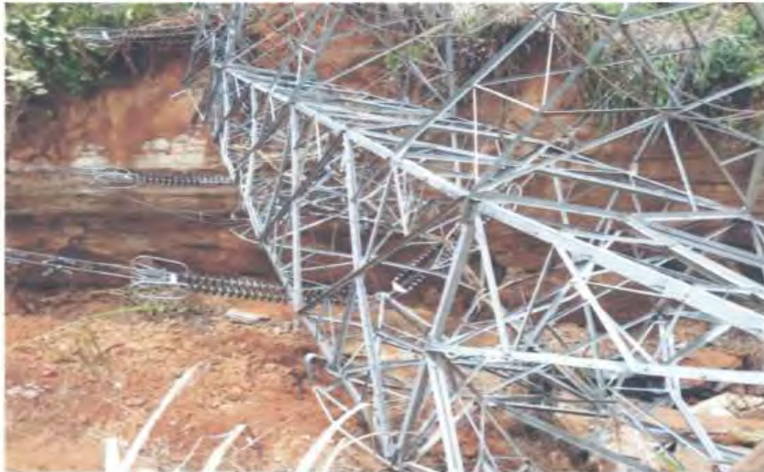
Collapsed tower no. 377 due to landslide
