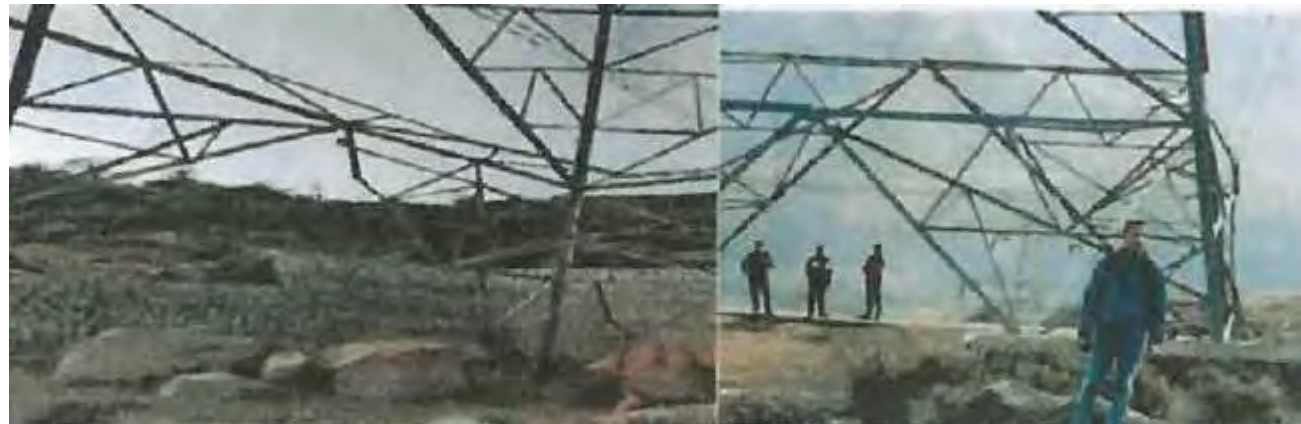
Bending of members of Tower at location no. 144
