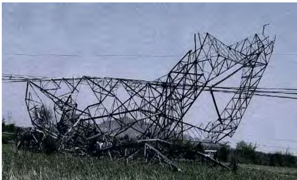
Tower at location No. 394 (72/1(TTA+3))
